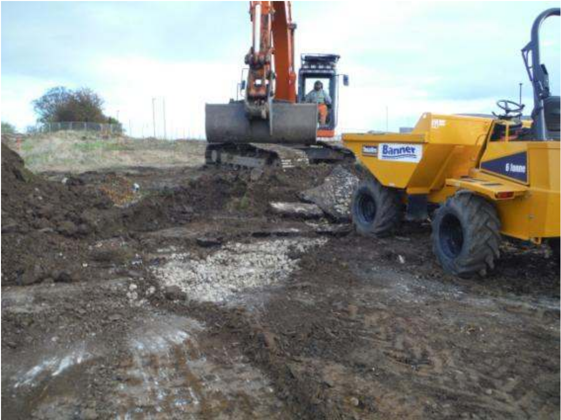
Plate 2. Exposing heavily disturbed deposits in the south-western area of the development area.
