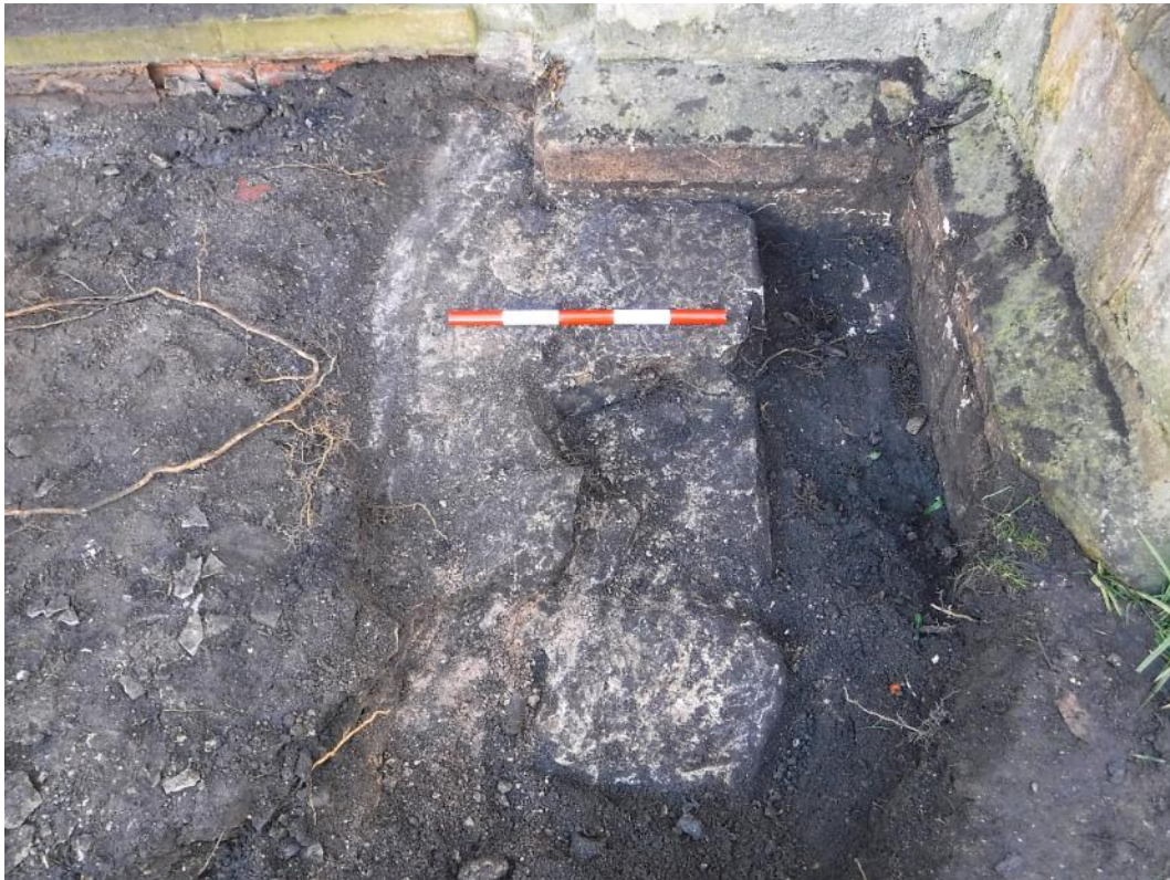
Plate 4 Footings and foundations for steps and threshold, facing southeast, scale unit 100mm
