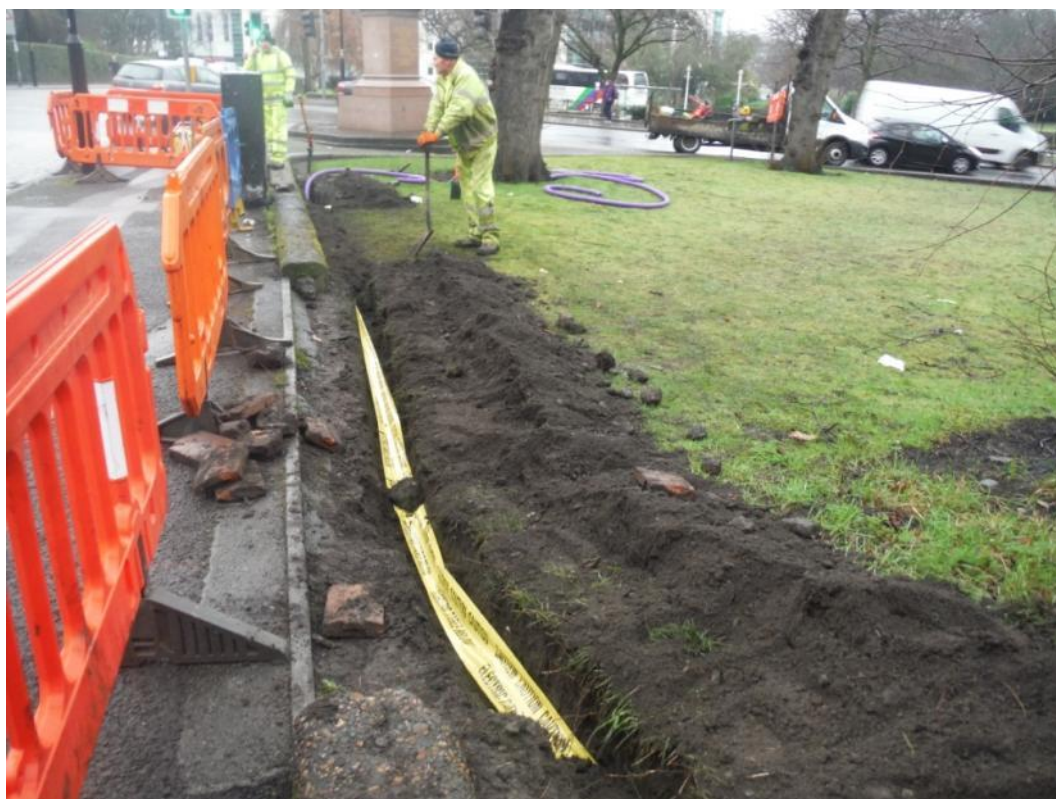
Plate 6. Ducting and electrical cable trench running into mains fuse box, facing west.
