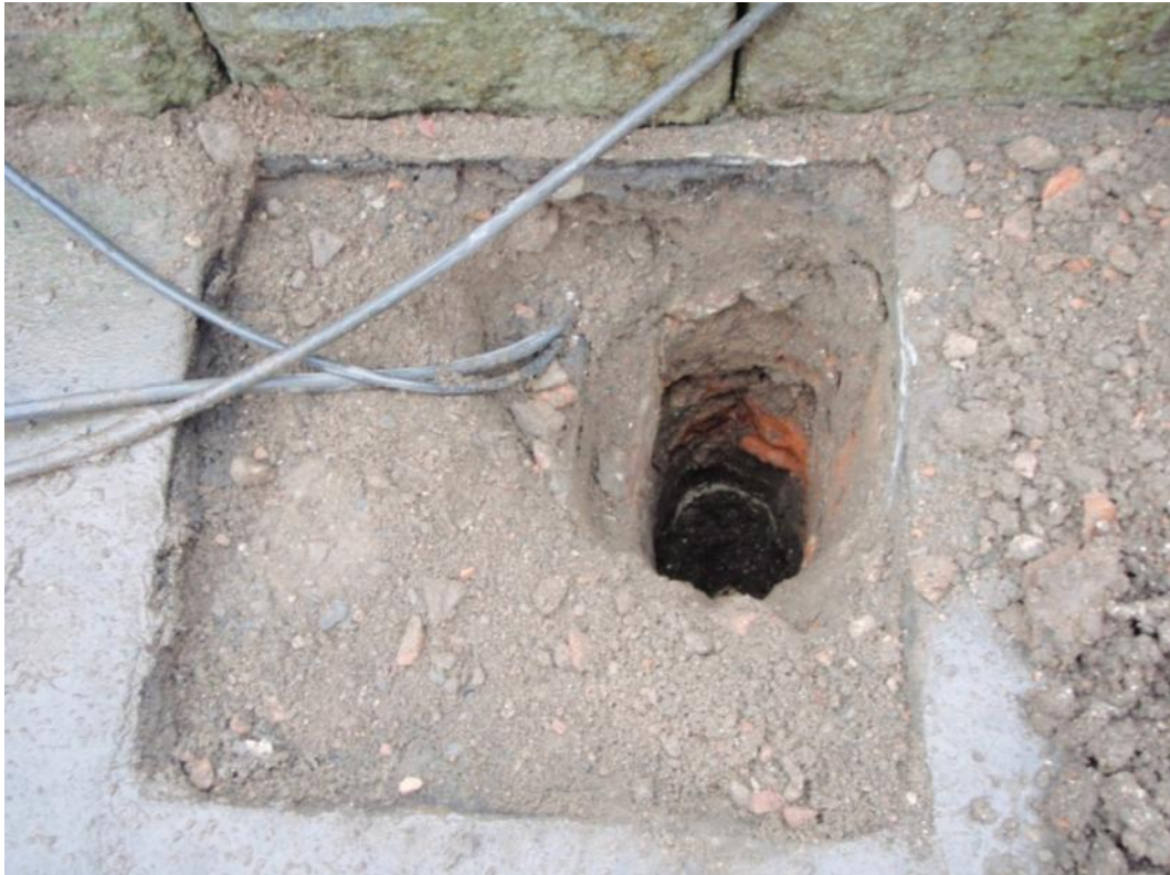
Plate 4. Existing lighting cable and 1m excavation slot for new lamp post, in south-east corner.
