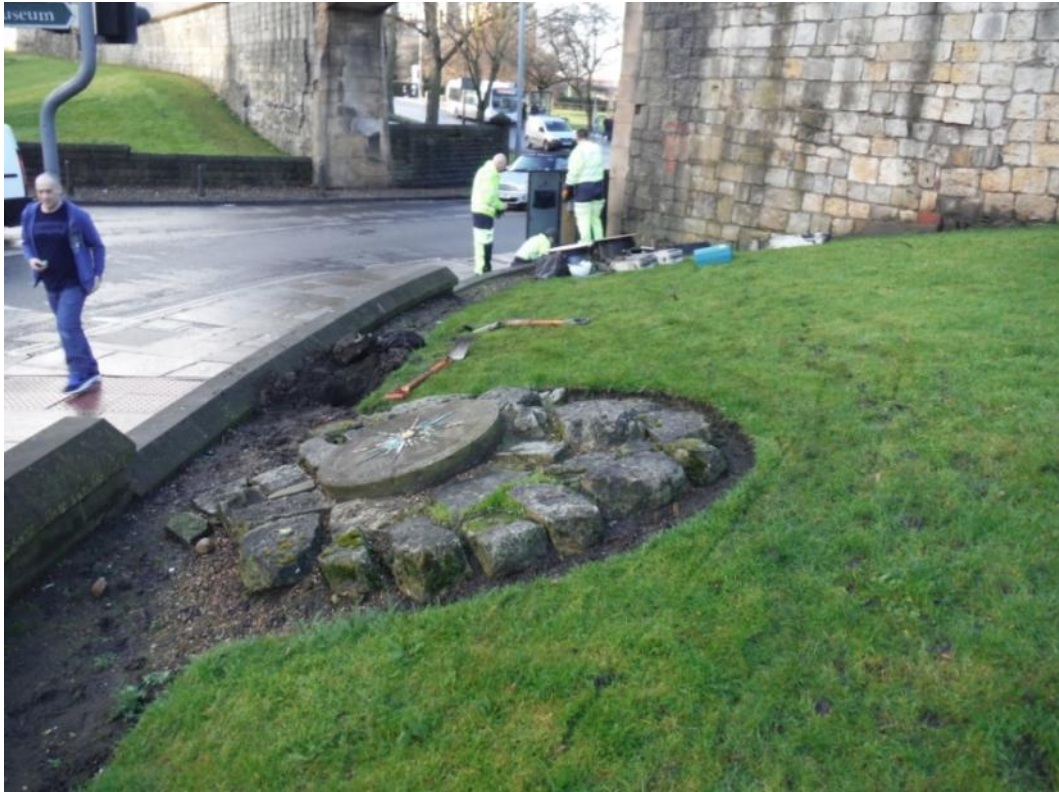
Plate 2. Lighting slot and cable running to fuse box, facing south-west.
