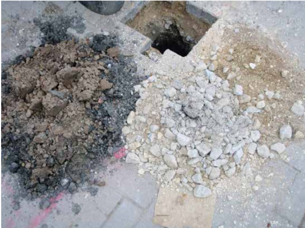
Plate 6: Borehole 1 (Arisings from the manual excavation of 0-1m, 1m depth deposits to the left)
