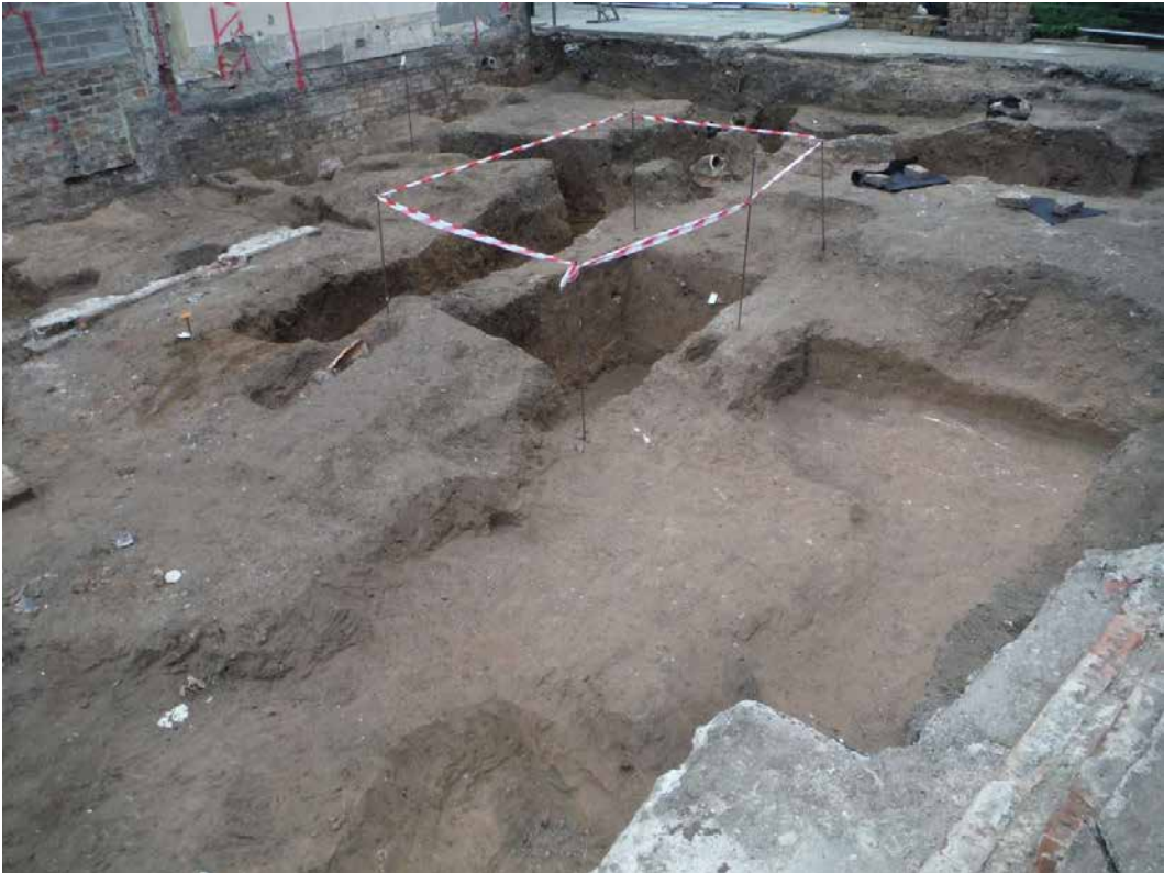
Plate 35 A deep intrusion (within the extent of the red and white barrier tape) relating to the late 20th century hotel extension. Looking W.
