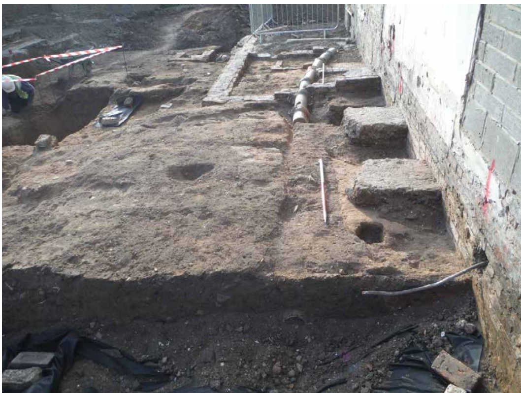
Plate 32 Ceramic drain pipe S3005 originally emerging from the SE corner of 147 Mount Vale, later made redundant with the instillation of drain S3004. Looking SE, 0.5m scale units.
