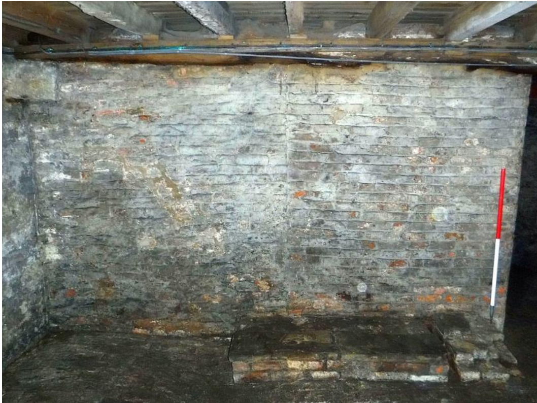
Plate 6 Partition wall and later addition to left, facing north-east, scale unit 500mm
