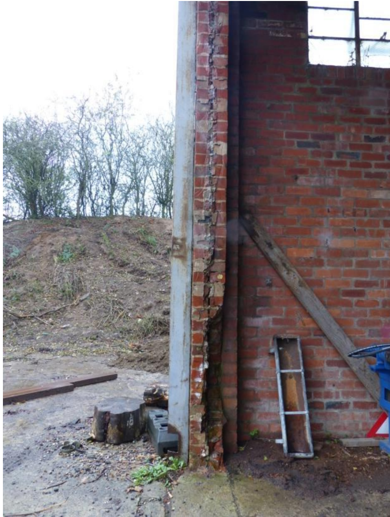
Plate 4: Damaged brickwork on the front elevation door opening, looking west
