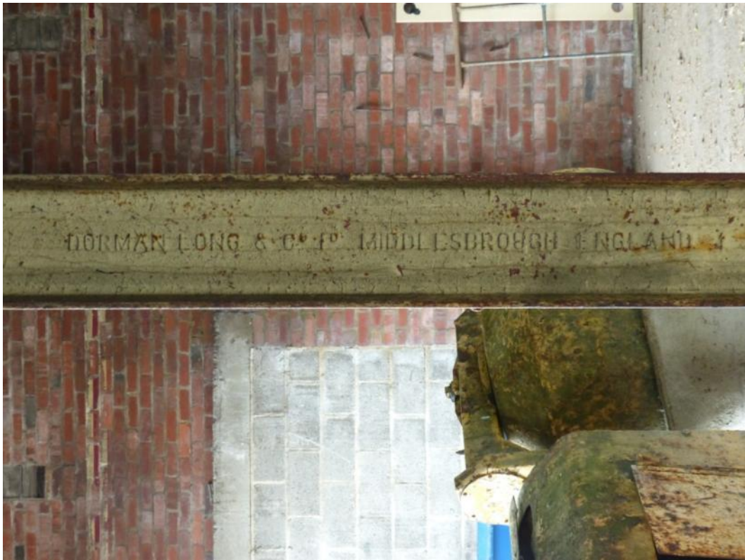
Plate 11: The raised lettering on the steel girders reading "DORMAN LONG & Co Ld MIDDLESBROUGH ENGLAND"
