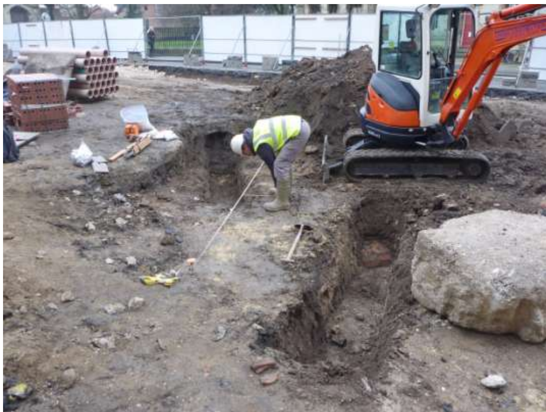
Plate 18 Trench E to left with initial excavation of Trench F to right, looking south east
