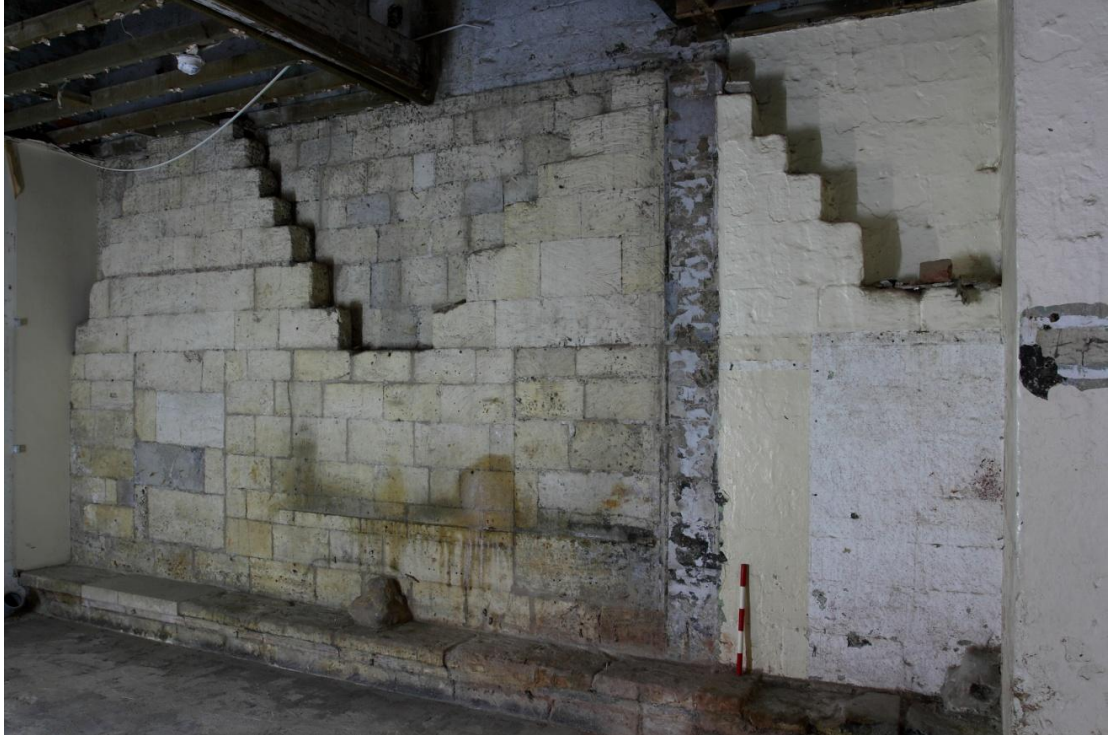
Plate 1 Easternmost elements of former range. Note shaft bases atop wall-bench and two blocked openings, looking SE
