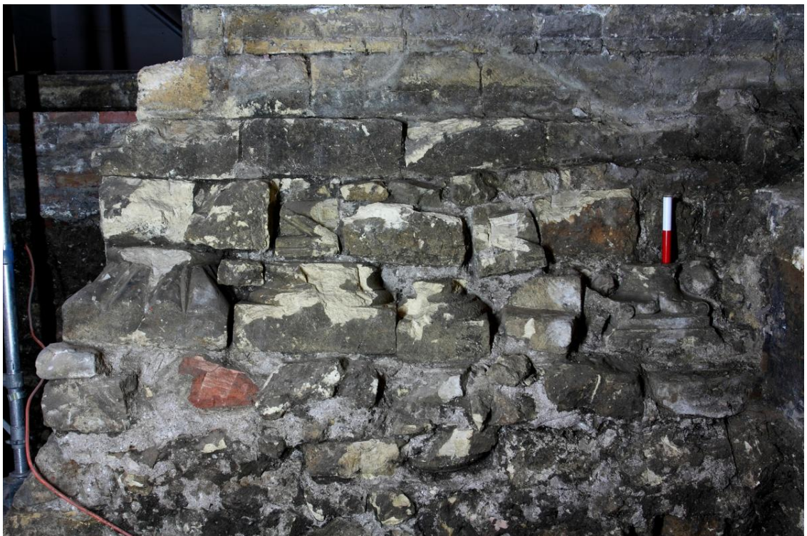
Plate 6 Detail of reused 12 th century masonry in 15 th century buttress footing, looking east
