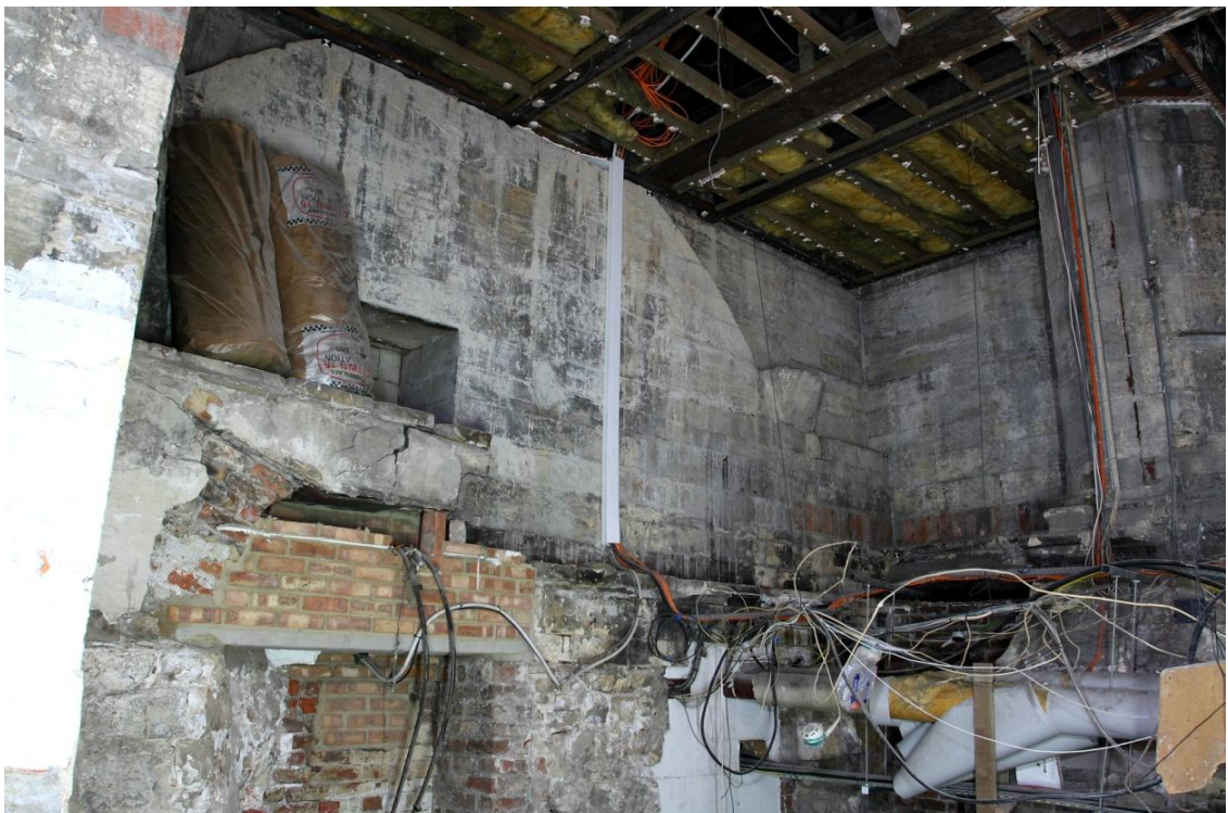
Plate 4 Westernmost elements of former range, north transept is to right, looking SW
