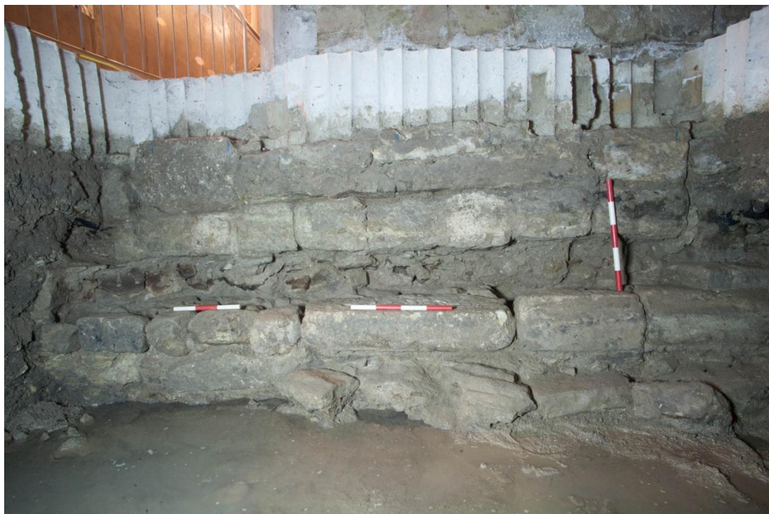
Plate 20 Elevation 2 (west facing) after removing the upper stones of 1067 (Image taken by Stuart Harrison)
