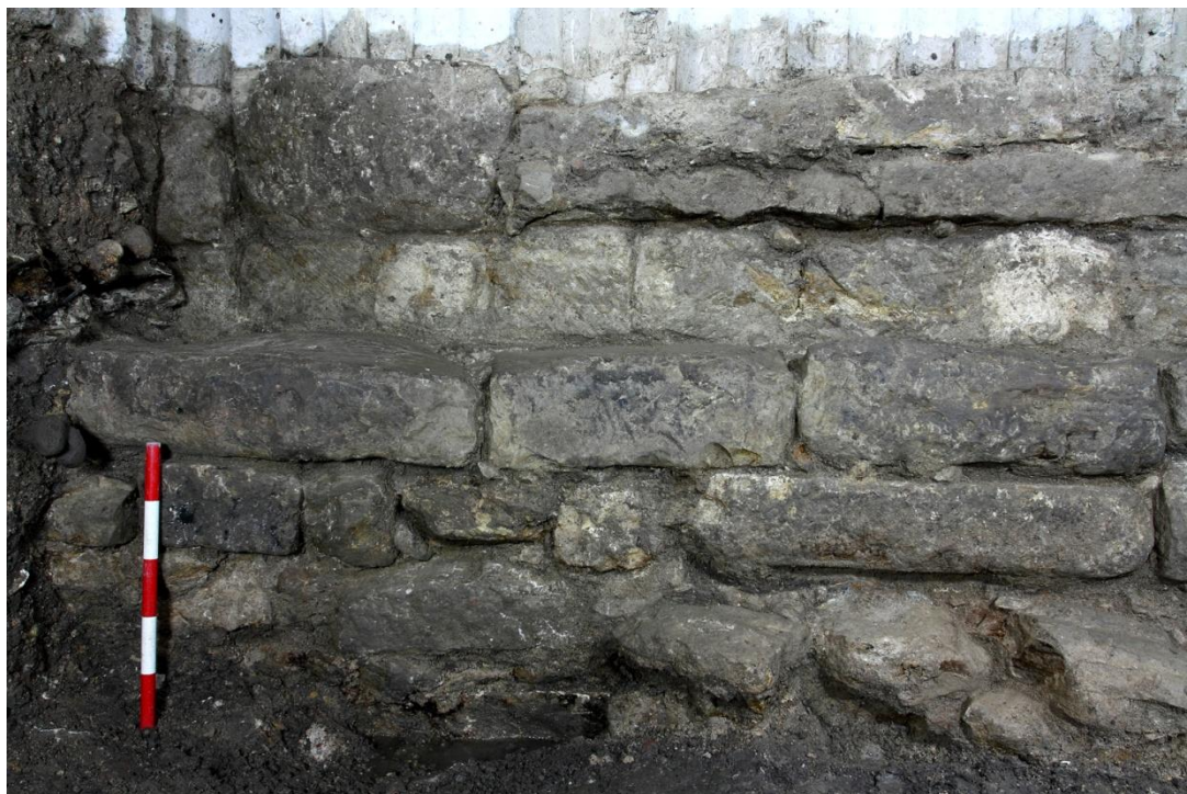
Plate 16 Northern end of elevation 2 (west facing) prior to removal of the projecting part of 1067, looking east.
