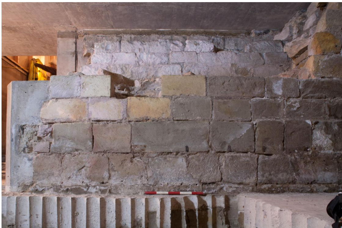
Plate 26 North end of west facing C13th South Transept arcade foundations, looking east (Image taken by Stuart Harrison)
