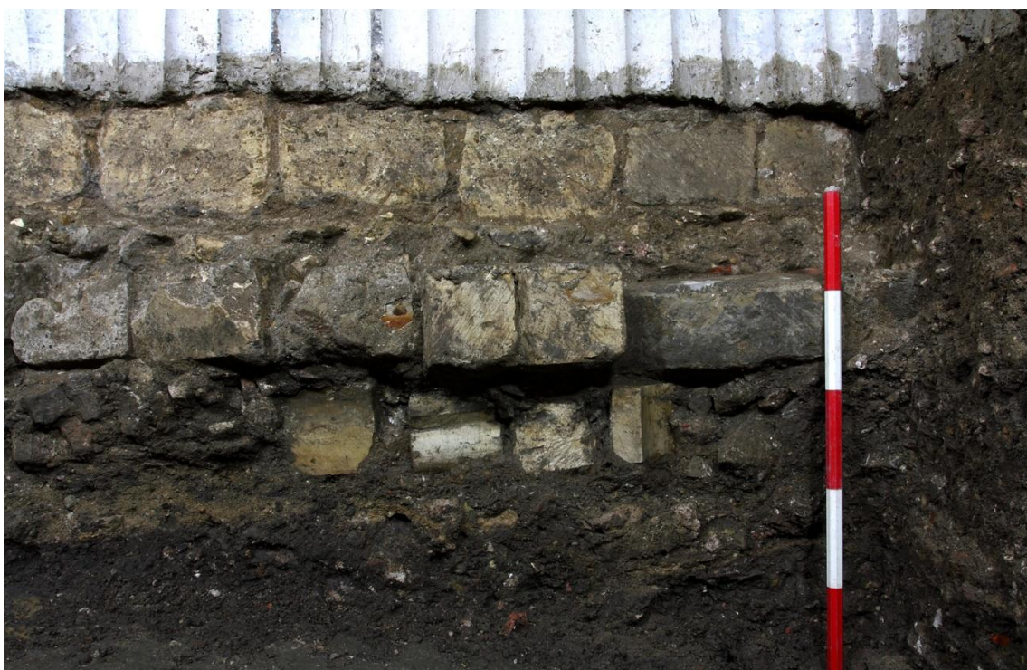
Plate 19 Northern end of elevation 4 (east facing) prior to removal of the projecting part of 1043, looking west
