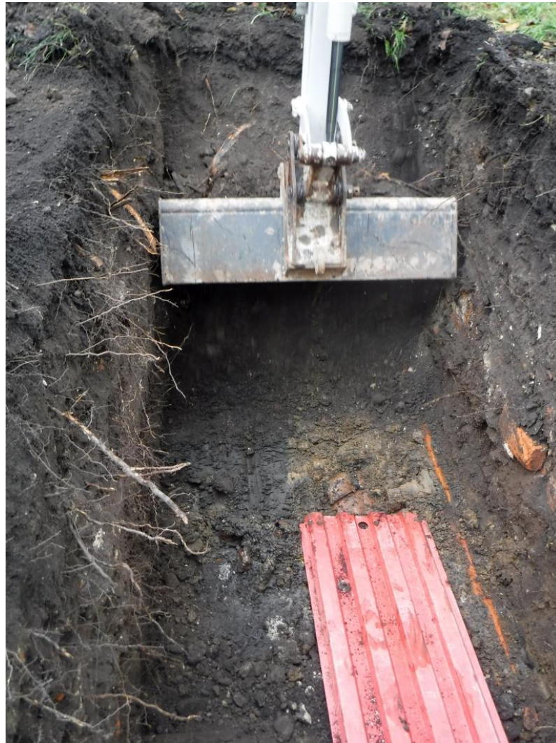
Plate 1 Trench 1 drain being repaired beneath shoring sheet and older culvert to the right, facing northwest
