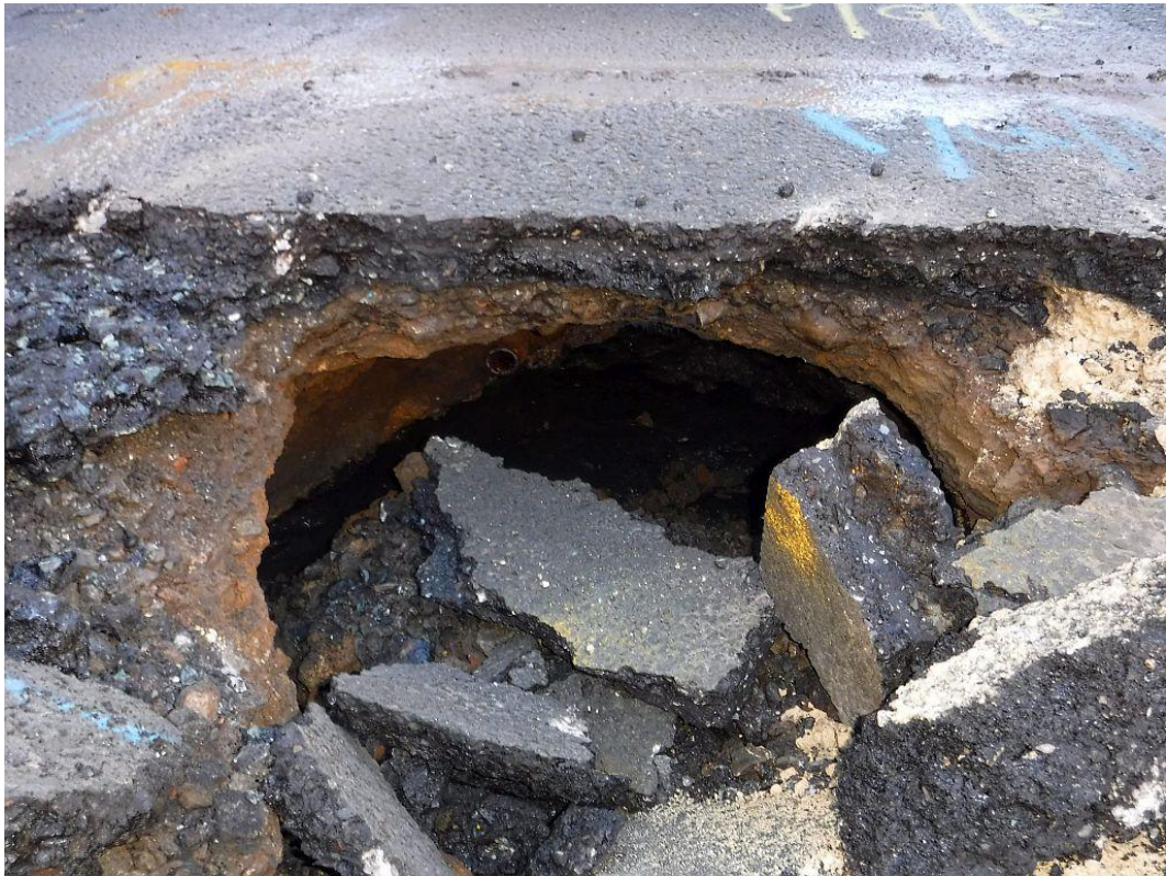
Plate 1 Sewer collapse, facing southwest
