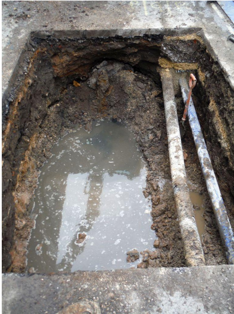
Plate 2 Sewer collapse extending lower in deposit sequence with contaminated liquid ingress, facing southwest
