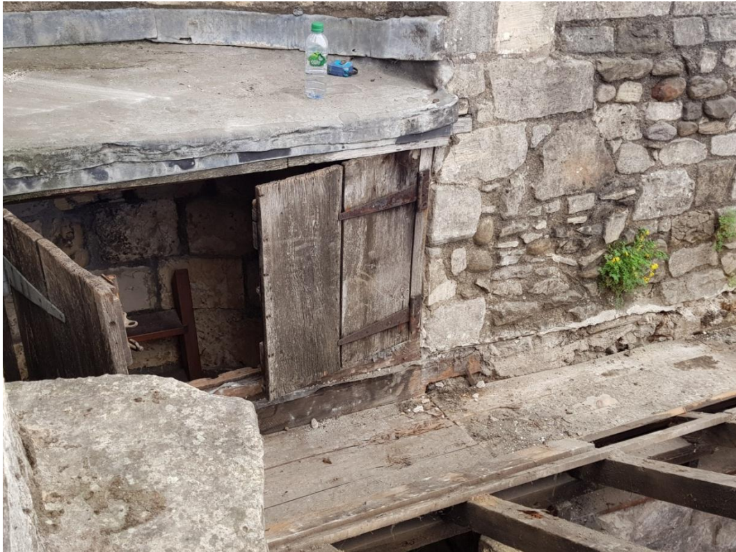
Plate 5 View of the hatch in the southwest bartizan providing access to the top of the roof and guttering, looking west
