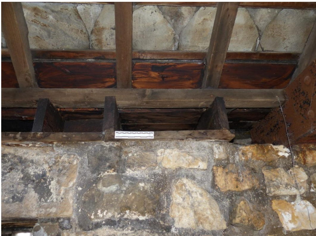
Plate 4 Timber joists supporting the guttering seen below the common rafters, looking west
