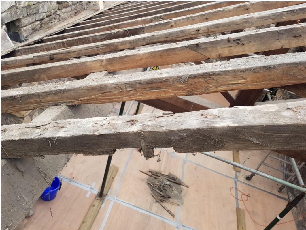
Plate 10 Detail view of the reused common rafters in the northeast corner bay, looking south
