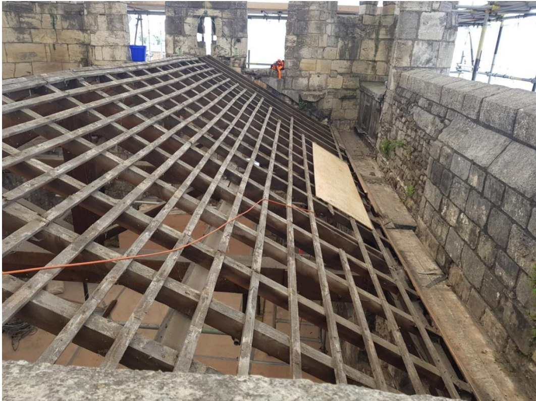
Plate 7 General view of common rafters and battens on the west half of the roof
