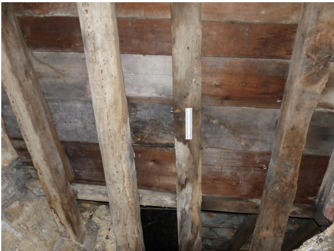
Plate 18 View of timber reused timber joist in east bartizan roof, looking up and west
