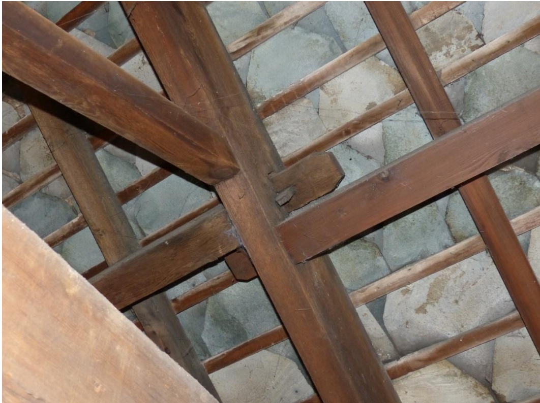
Plate 11 Detail view of the purlins overlapping and running through the principal rafter
