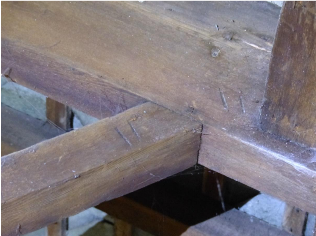
Plate 13 Detail of carpenter's marks on the Truss 2 where the strut and principal rafter meet
