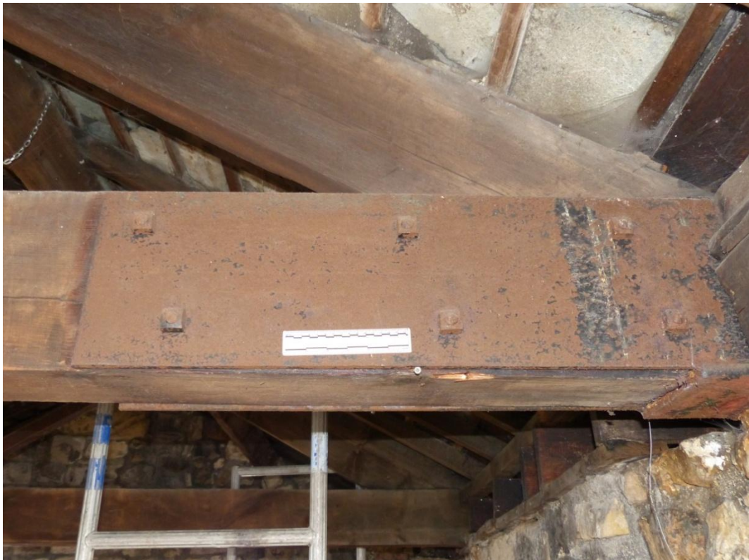
Plate 12 Detail view of the steel jacket supporting the west end of Truss 1
