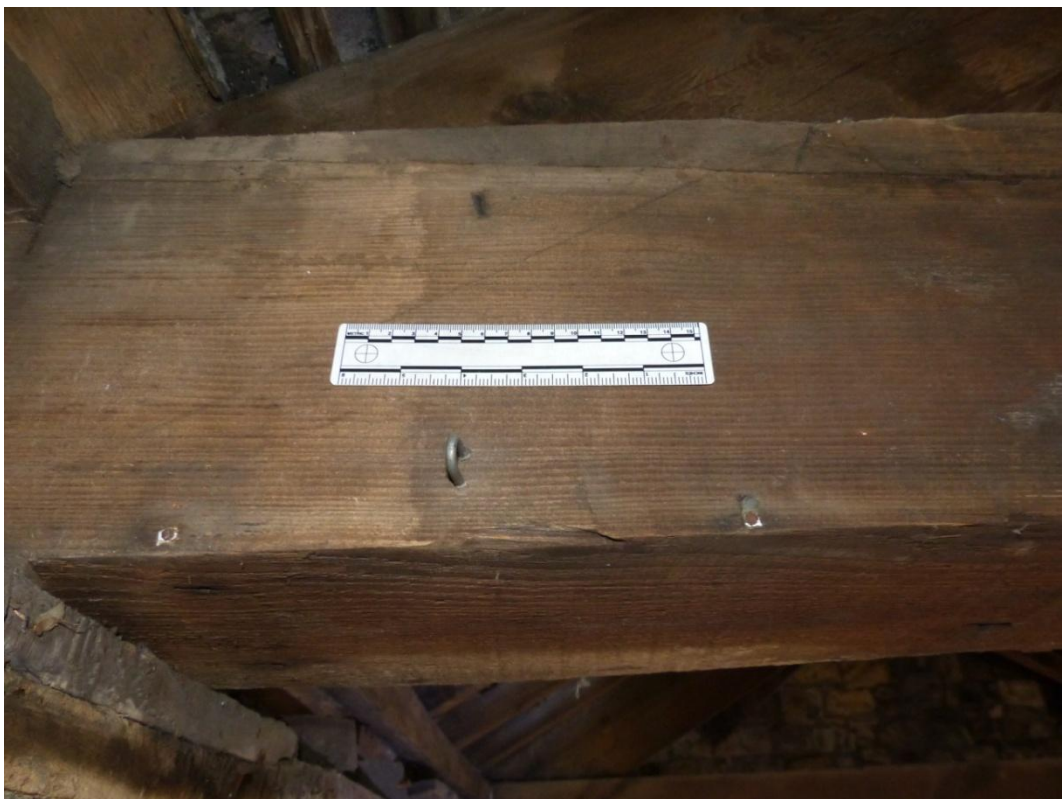
Plate 14 Detail view of the purlins overlapping and running through the principal rafter
