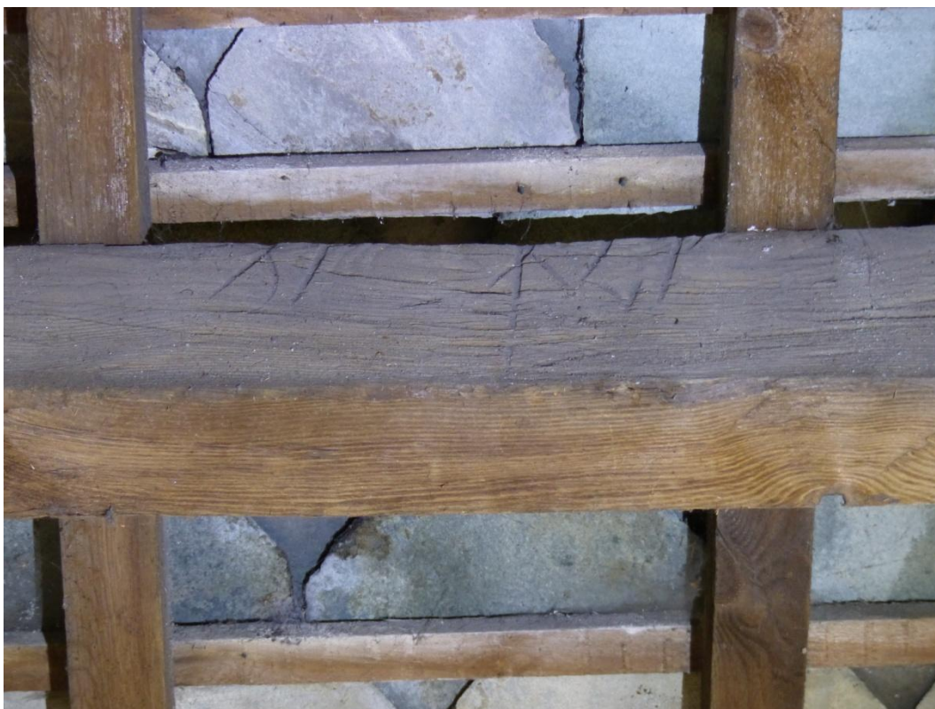
Plate 15 Detail view Baltic timber marks on the west purlin in the central bay
