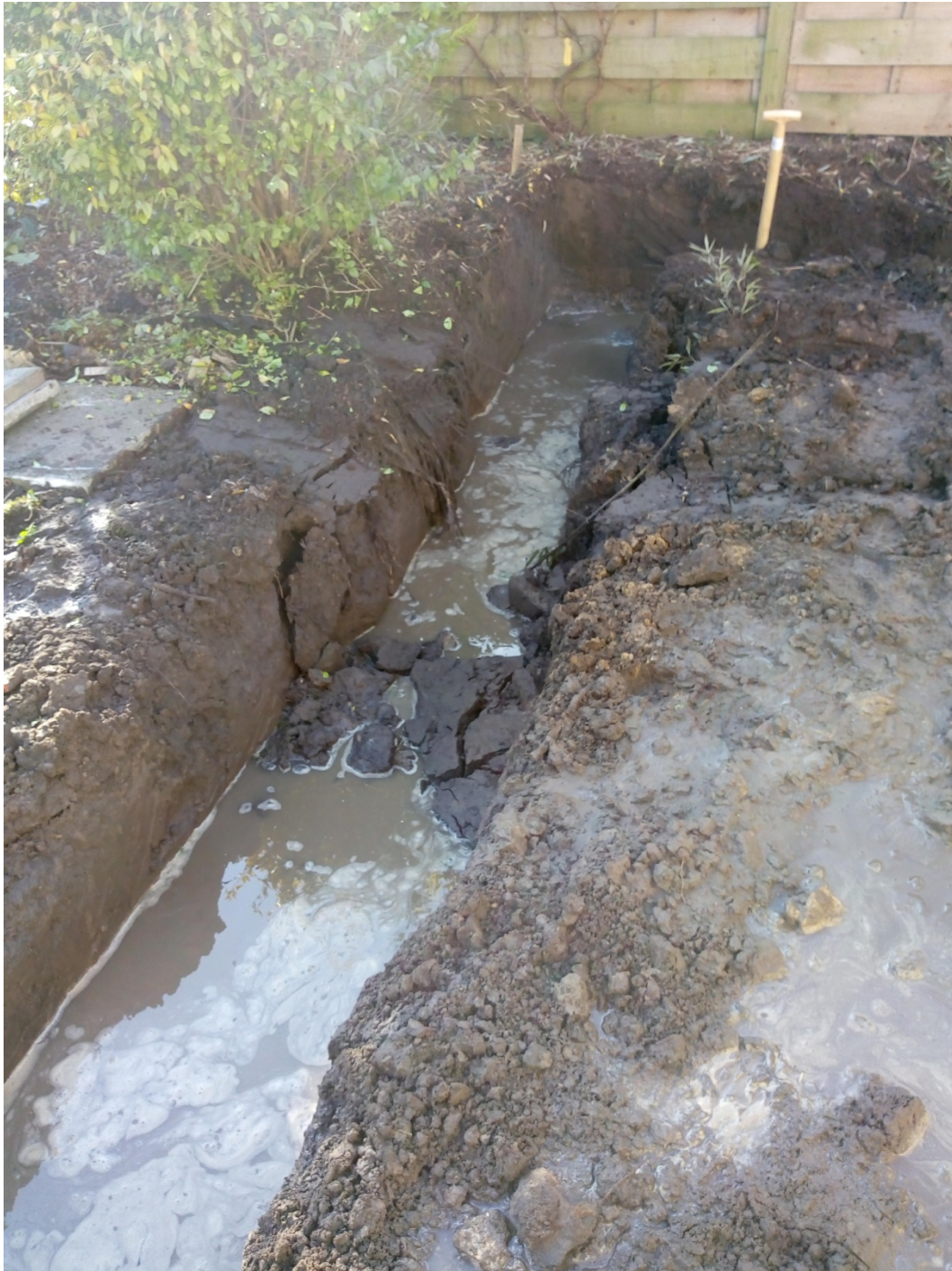
Plate 2 Foundation trench to rear of site filled with ground water, view south.
