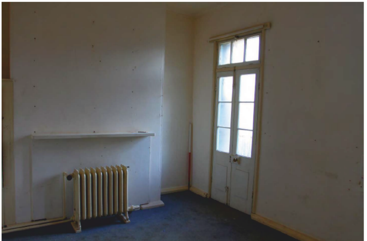
Plate 42 First floor parlour in the Extern with door onto balcony, looking northeast.
