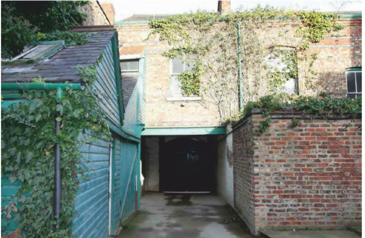
Plate 3 Partial view of the southern elevation of the Lodge from the rear courtyard, looking north. Includes details of the carriageway, private stair and internal walls.
