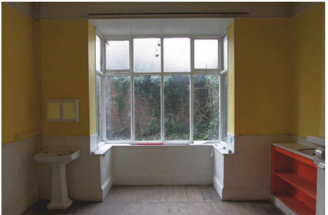
Plate 12 View of the bay window, a 20th century addition, in the rear parlour of the Lodge, looking south
