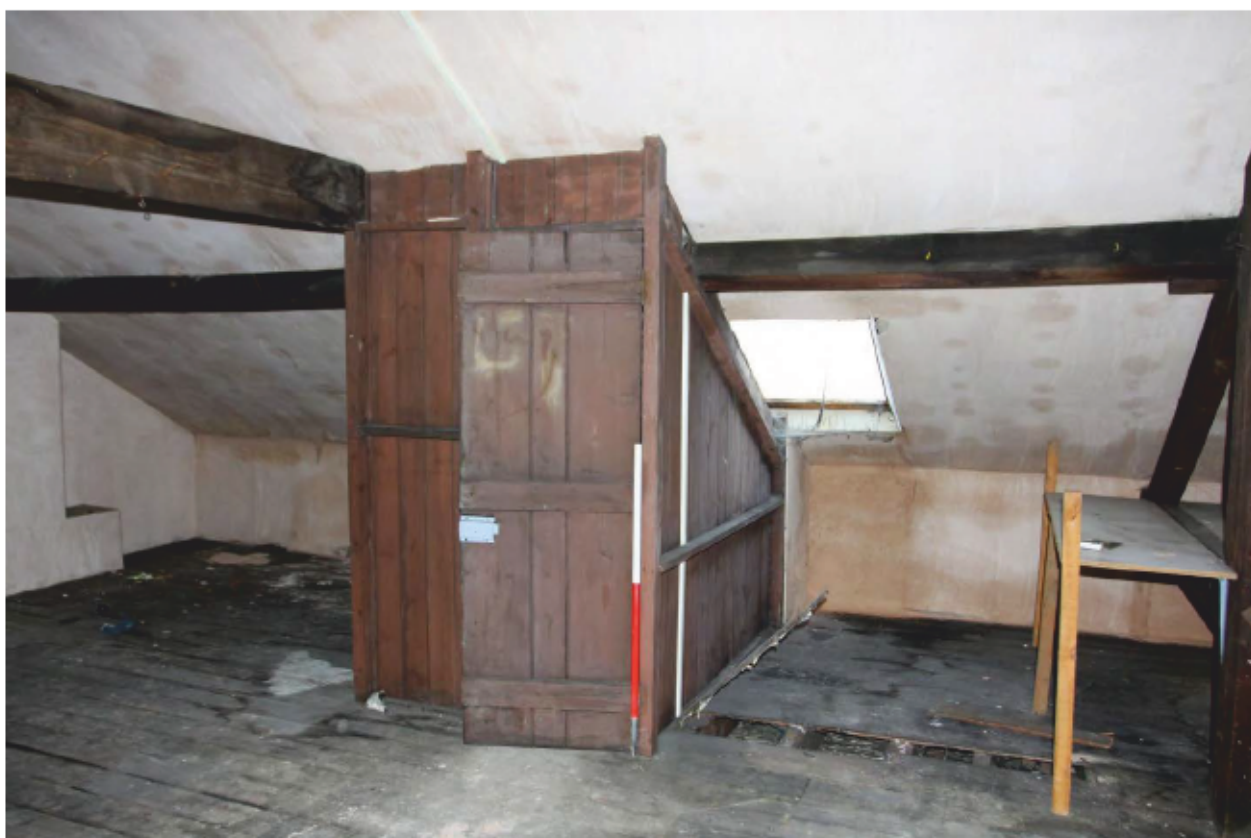
Plate 18 Loft space within the Lodge including top of staircase, looking north west.
