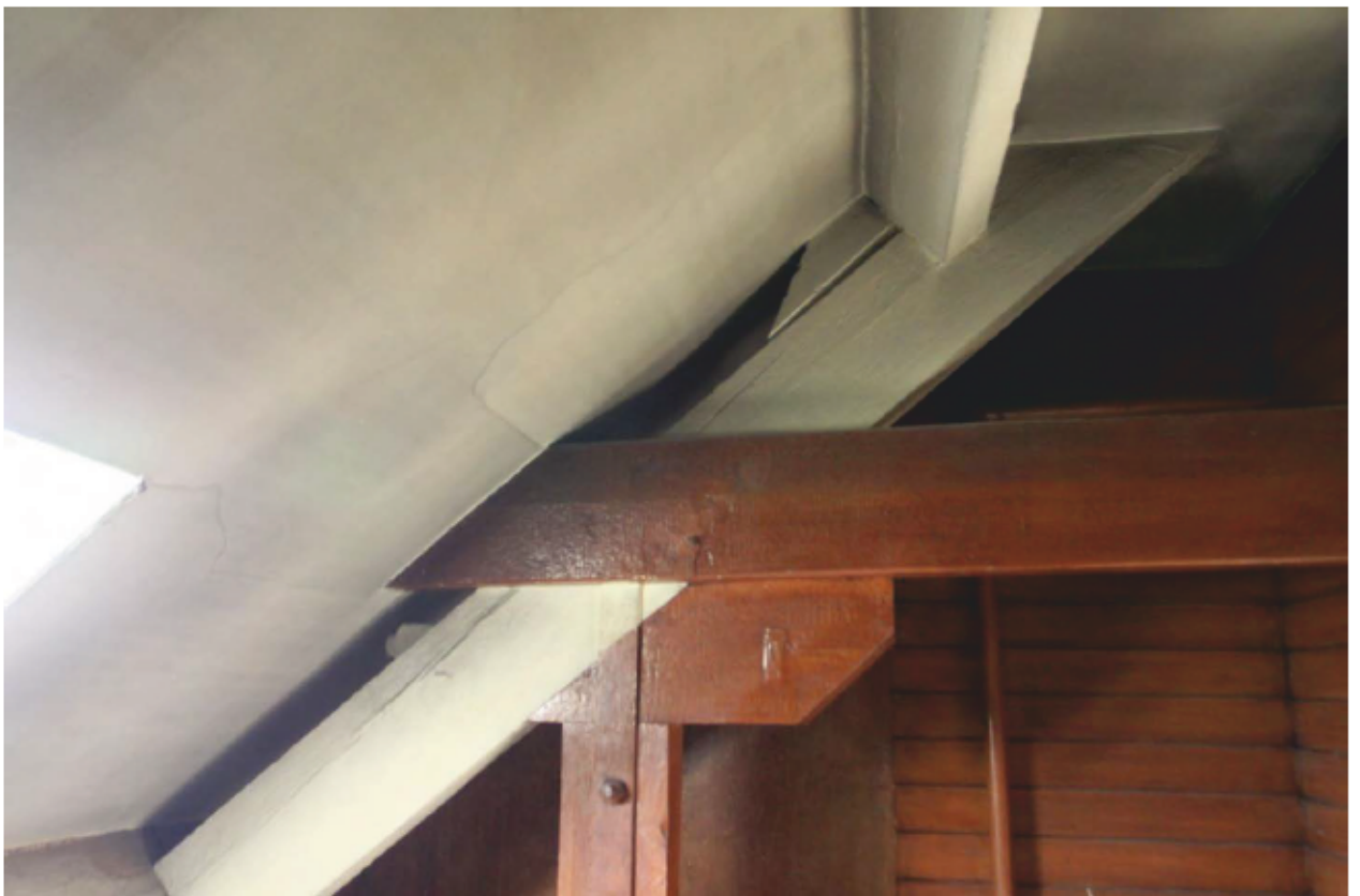
Plate 44 Alterations to the straining beam of the queen post roof in the Extern.
