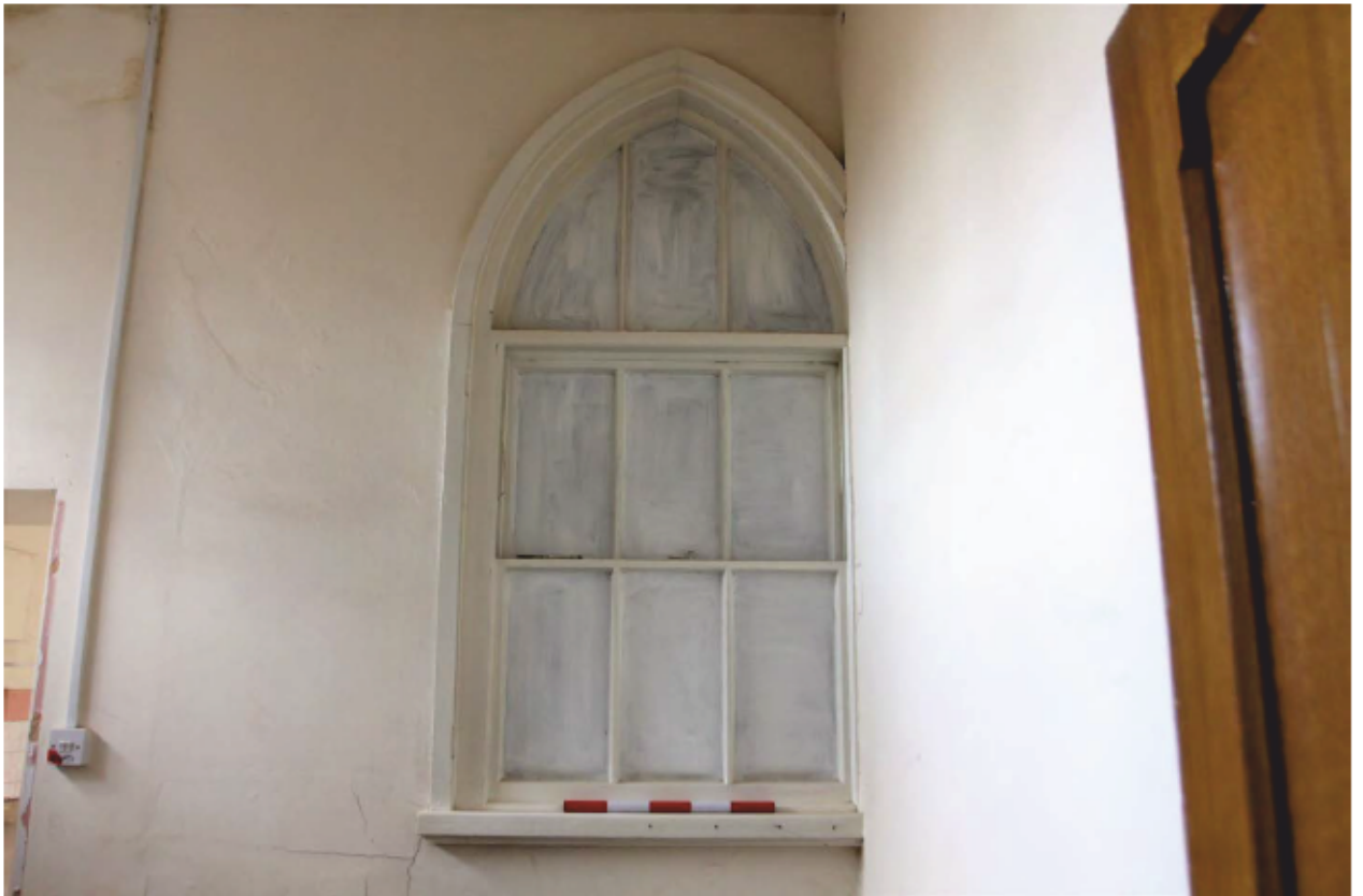
Plate 39 Internal view of the blocked up window on the eastern elevation, looking east.
