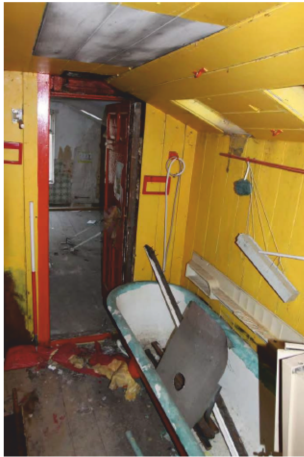
Plate 25 View of the 20th century bathroom and loft conversion within the single storey extension, looking east.
