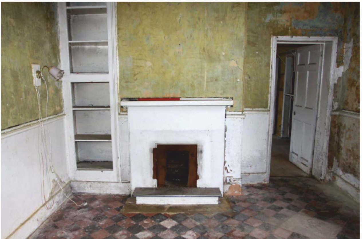
Plate 14 Rear ground floor bedroom of the Lodge with a fireplace, cupboards, dado rail and original floor, looking east. Flanking the fireplace to the right is the entrance into the single storey extension.
