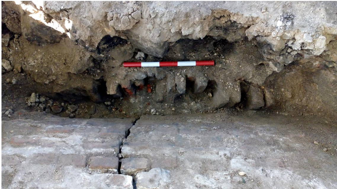
Plate 2 Junction of small room brick vault, at the top of the plate, with the main brick vault arch at bottom of plate
