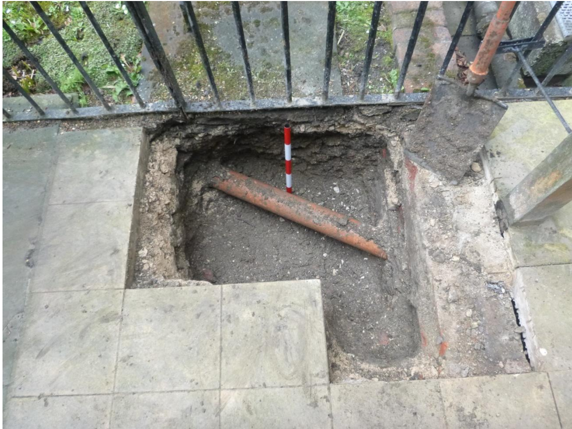
Plate 2 Post-excitation photograph of trench showing ducting and brick chamber (right). Scale: 0.5m
