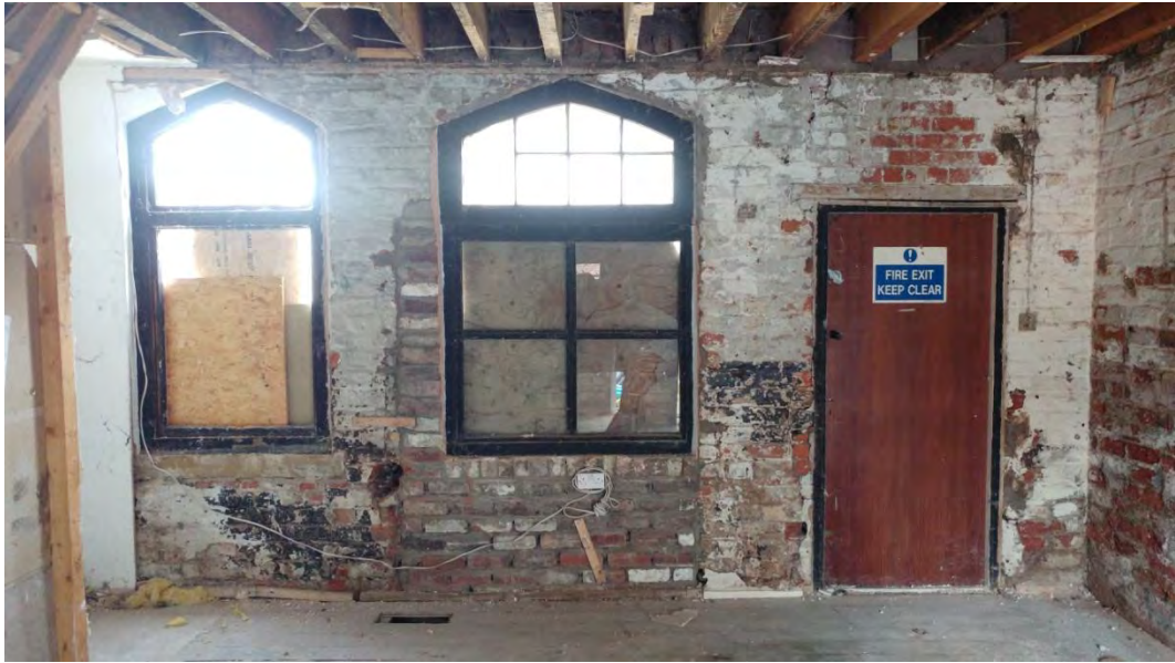
Plate 20 East wall of west coach house showing evidence of former door opening, looking east
