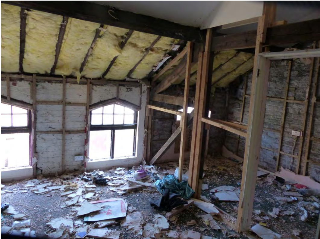
Plate 24 First floor east wall and roof truss of west coach house, looking south-east
