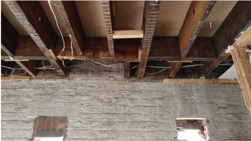
Plate 22 Possible feed drops in south room of west coach house, looking west
