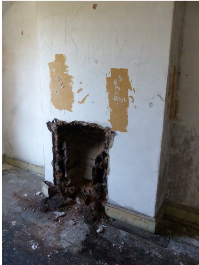
Plate 44 Detail of removed fireplace in first floor bedroom of cottage, looking north-west
