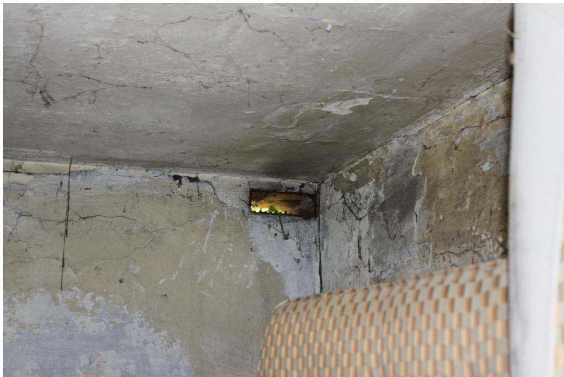
Plate 17 Gap in south-eastern corner of Building 2, view south-east.
