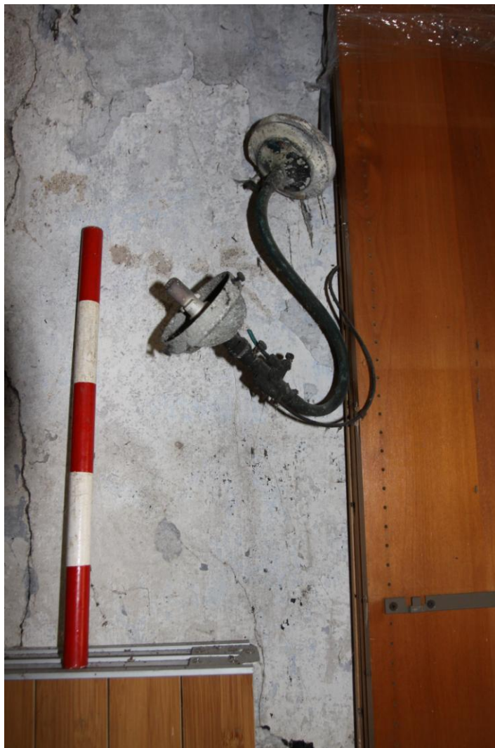
Plate 15 Gas light fitting in Building 2, view west.
