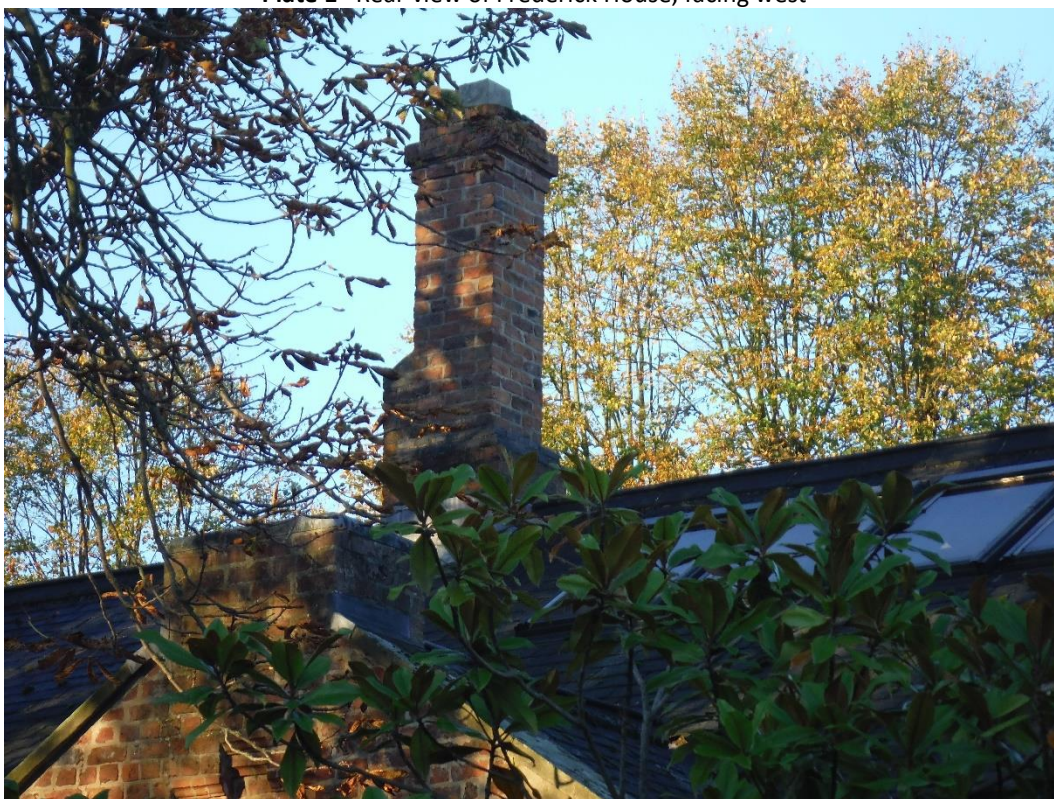
Plate 2 View of one of the Chimneys to the south of 'The Guard House' building facing west
