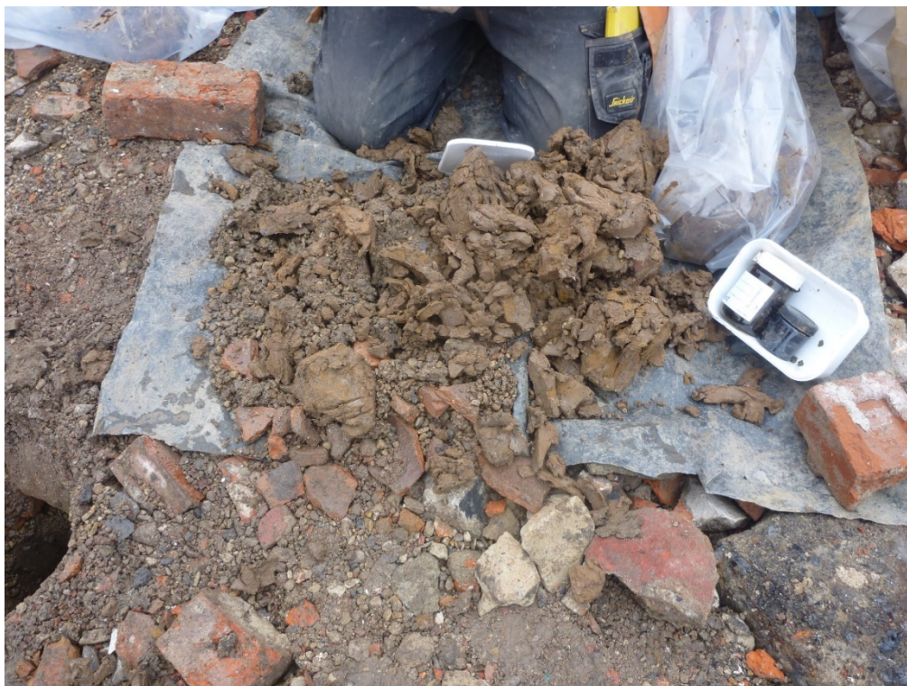
Plate 8 First metre of BH03, hand excavated. Frequent CBM visible in rubble/demolition deposit (C300) and gravel from drain bedding material (C301).
