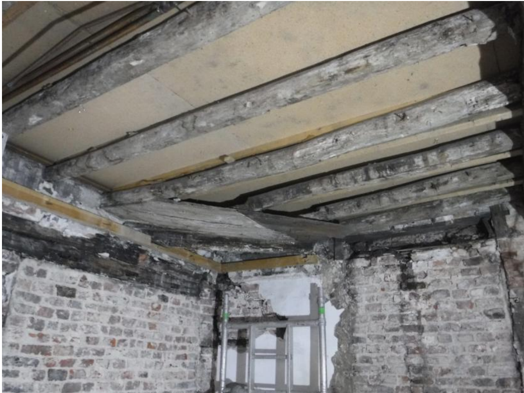
Plate 11 Planks attached below joists in the southern corner of the ground floor ceiling, facing south
