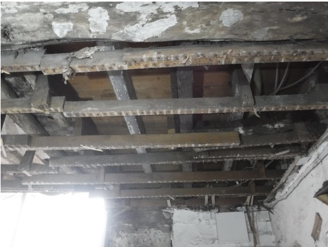
Plate 8 Reinstated 19th century ceiling battens and hangers across repaired section of ground floor ceiling in northern corner, looking north-west
