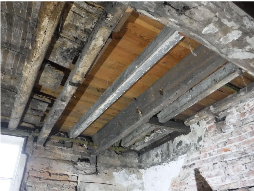
Plate 6 20th century joists inserted at north end of the ground floor, note the deteriorated early floor boards to left of shot, facing north
