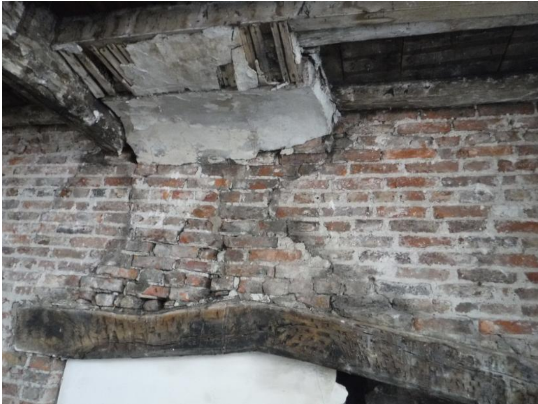
Plate 17 Support for first floor fire place above the north-western ground floor fire place, facing south-west
