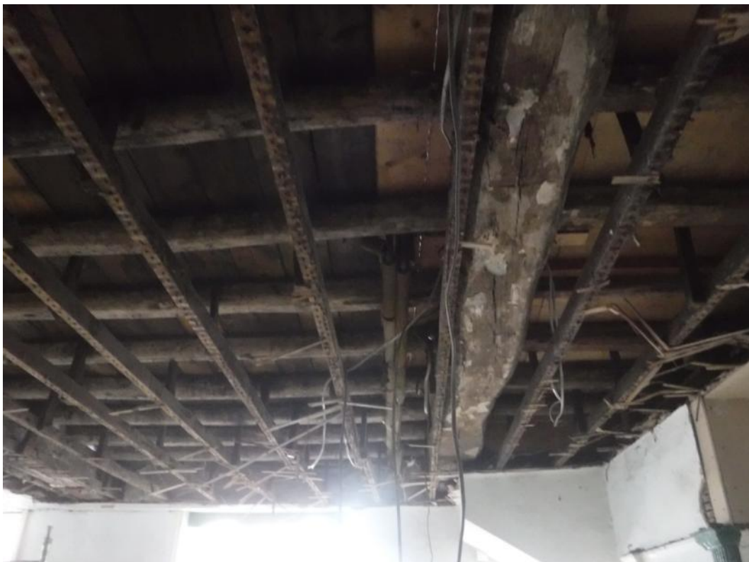
Plate 4 Battens and joist hangers used to support the 19th century lath and plaster ceiling, facing north-east
