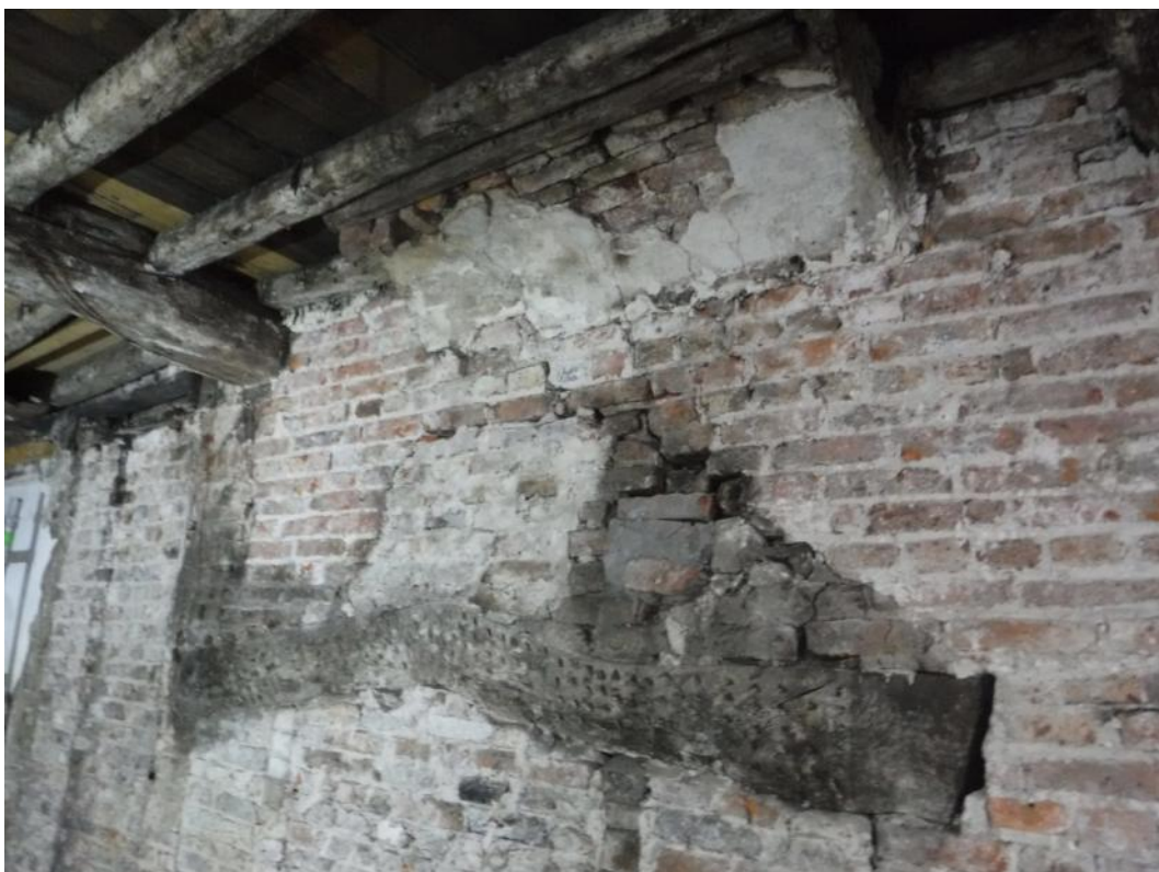
Plate 18 Support for first floor fire place above the south-eastern ground floor fire place, facing south
