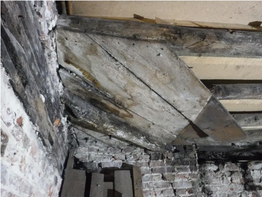
Plate 13 Detail of planks in southern corner of ground floor ceiling, facing south-west
