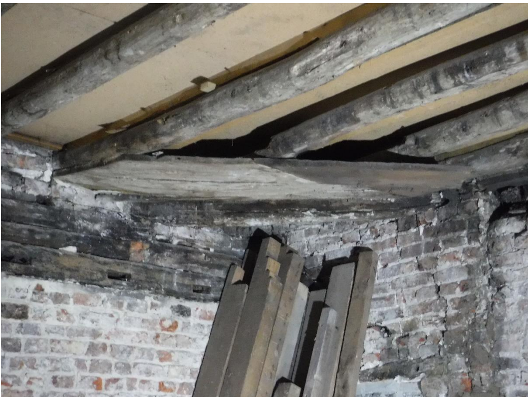
Plate 14 Detail of planks in southern corner of the ground floor ceiling, note the recesses on the upper part of the two joists running above the middle of the planks, facing south
