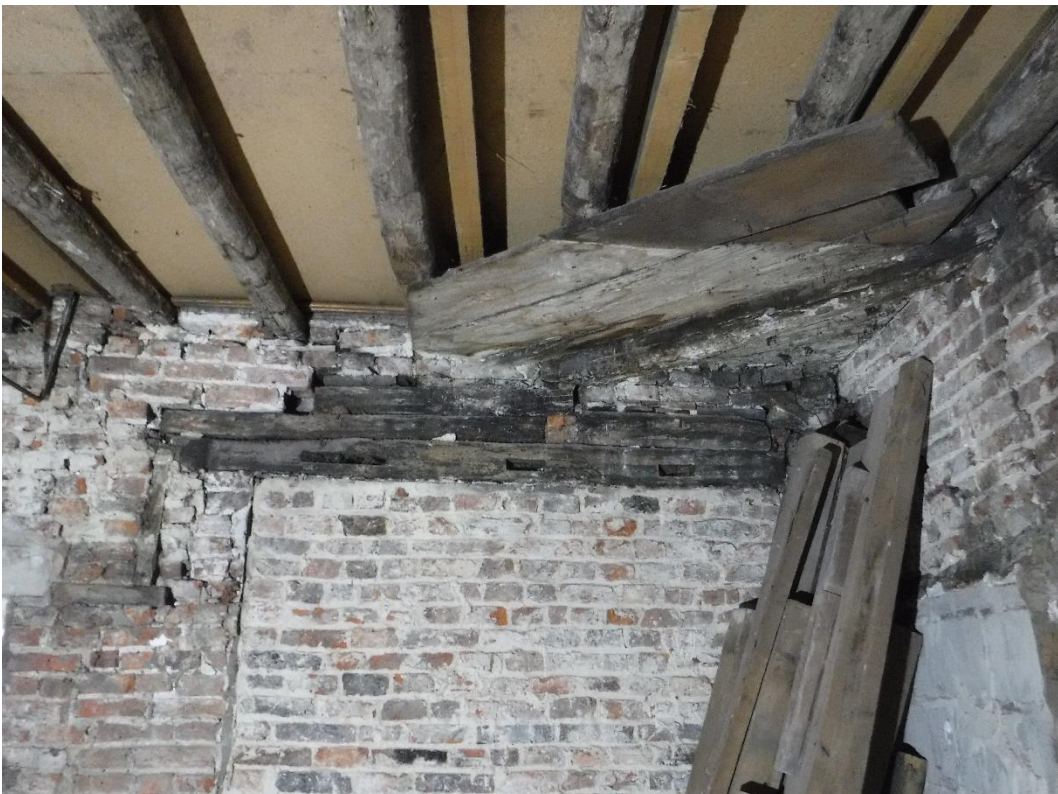
Plate 12 Planks attached to underside of joists in southern corner of the ground floor ceiling, facing south-east
