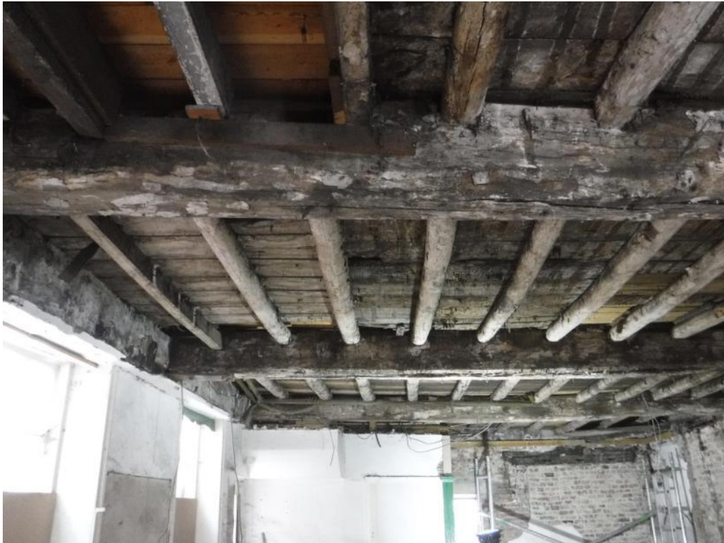
Plate 9 Exposed 17th/18th century beams and joists with floor boards of the first floor above, facing south-west
