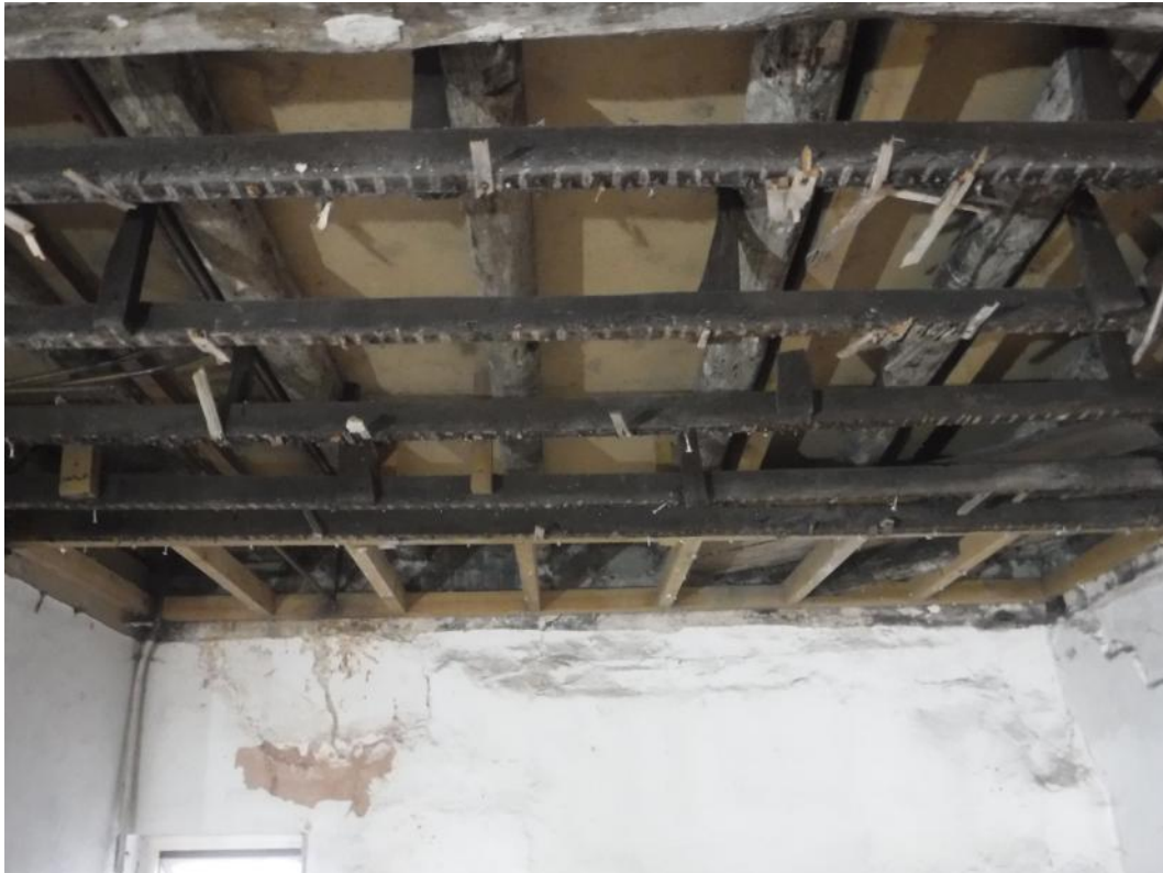
Plate 5 Modern battens alongside their 19th century equivalents at southern end of the ground floor ceiling, facing southeast
