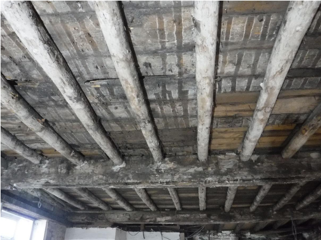
Plate 15 Traces of early lath and plaster ceiling visible on the underside of early first floor floor boards, facing south-east
