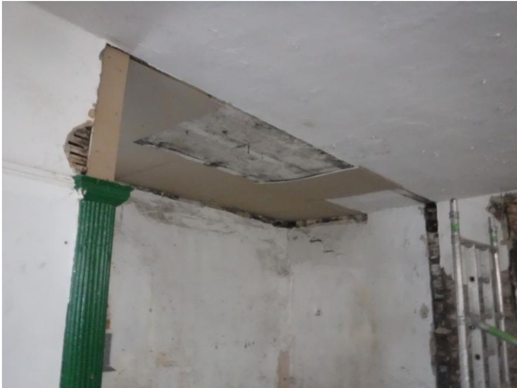
Plate 3 Modern repair to ground floor ceiling in recess at southern end, facing south
