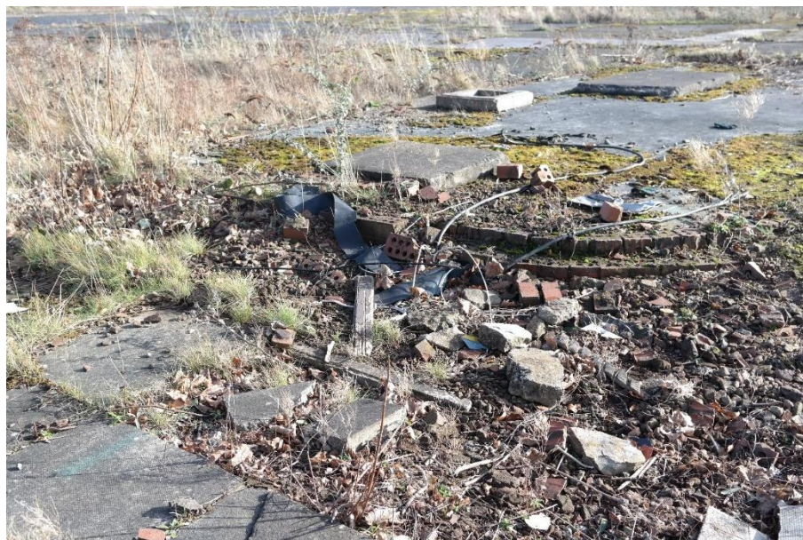
Plate 30 Debris on the building plinth of Zone D facing south-east
