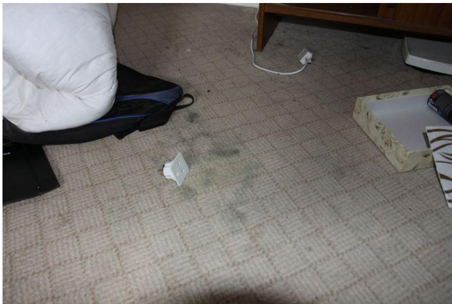
Plate 116 Room V the mouldy carpet
