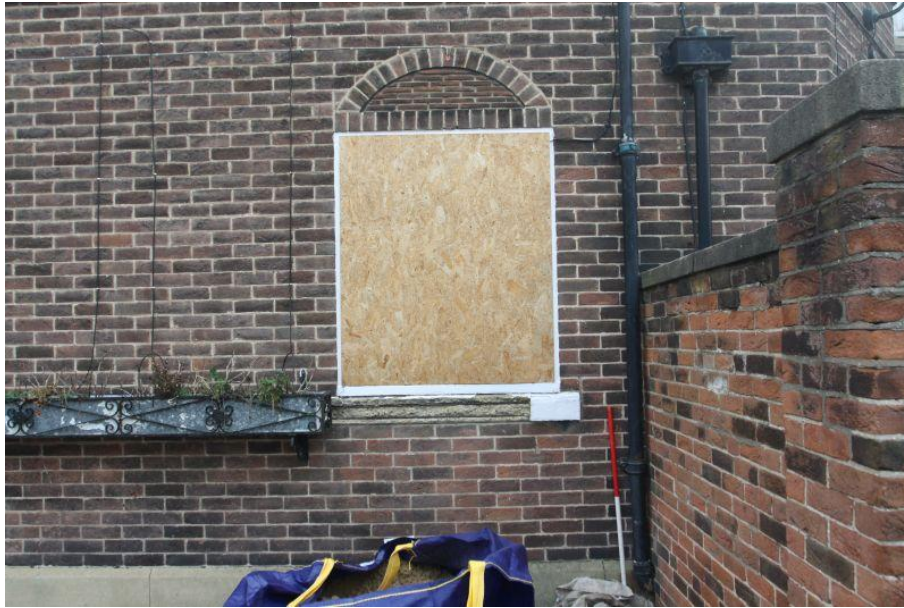
Plate 20 The decayed window sill on the south-western elevation, facing north-east
