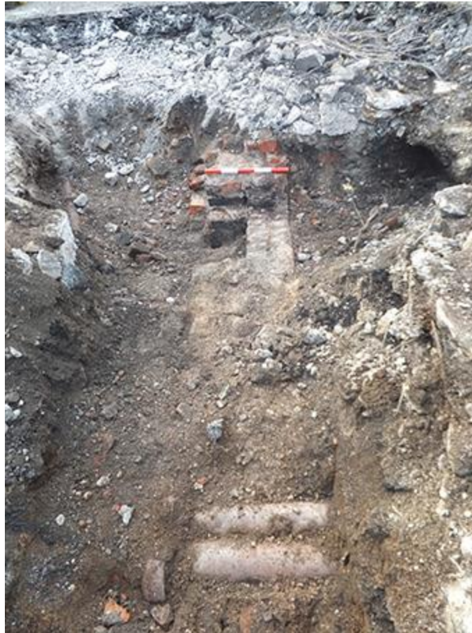
Plate 1 Test Pit 1. Modern services and elements of buildings formerly fronting Fossgate. Facing south-west, 0.1m scale units
