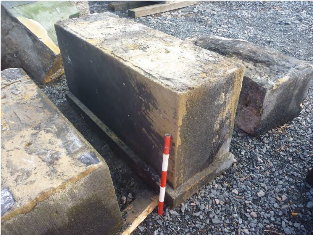
Plate 17 Example of masonry from lower course of the original abutments and pier with visible step out. Dated to 1845
