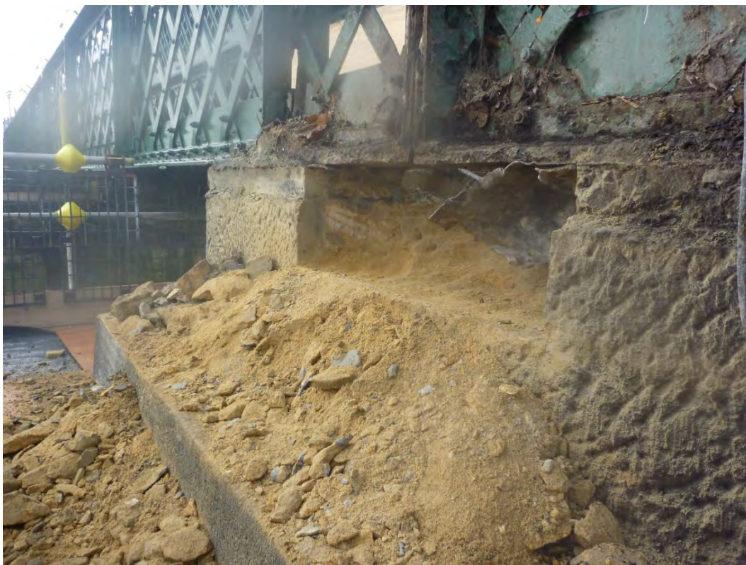
Plate 15 Removal of masonry from central pier and drilling into the pier in order to install the hydraulic system to raise and remove the footbridge
