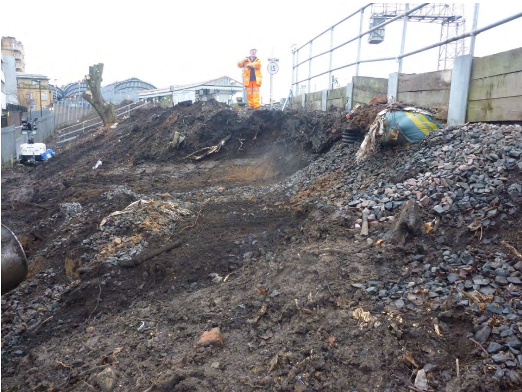
Plate 4 Overview of excavated step in the top of the embankment for sheet piling
