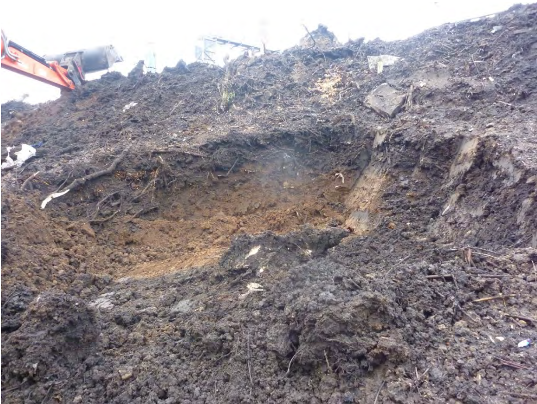
Plate 7 Representative section showing the greater depth of topsoil closer to the bridge
