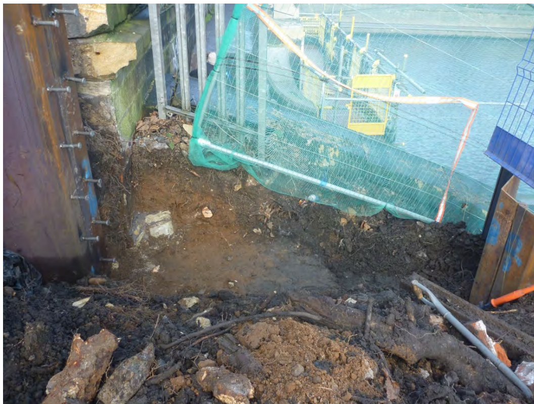
Plate 9 Section against existing masonry wingwall which illustrates the sloping deposits towards the embankment
