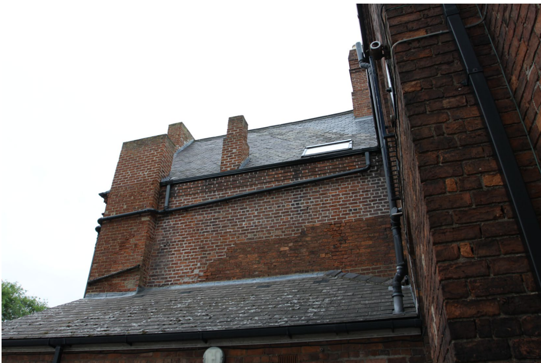
Plate 28 Roof light visible in south rear elevation of 210 Fulford Road, view north
