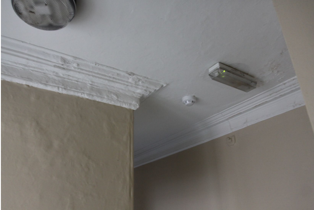
Plate 13 Damp in Bedroom 6
