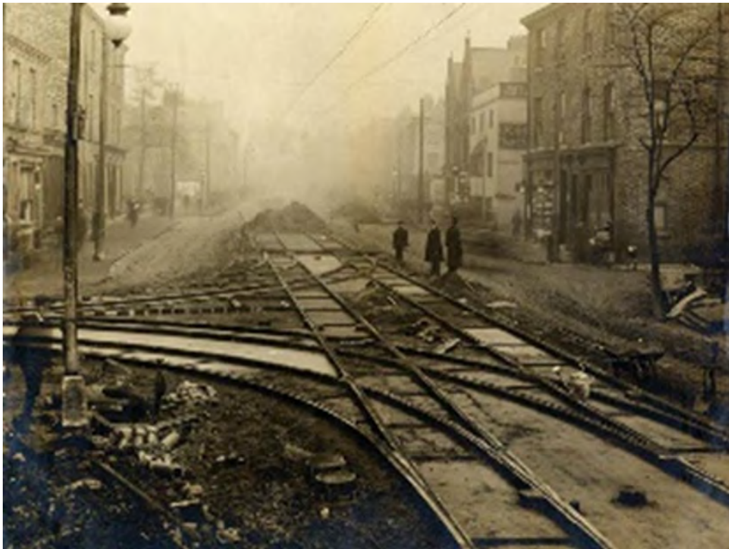
Plate 1 Looking towards Micklegate Bar in 1909 as new electric tram-lines are being laid.
