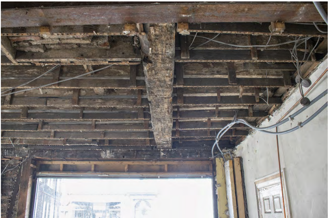
Plate 20 Original beam and joist timber floor with remains of lath-and-plaster timber sub-ceiling.
