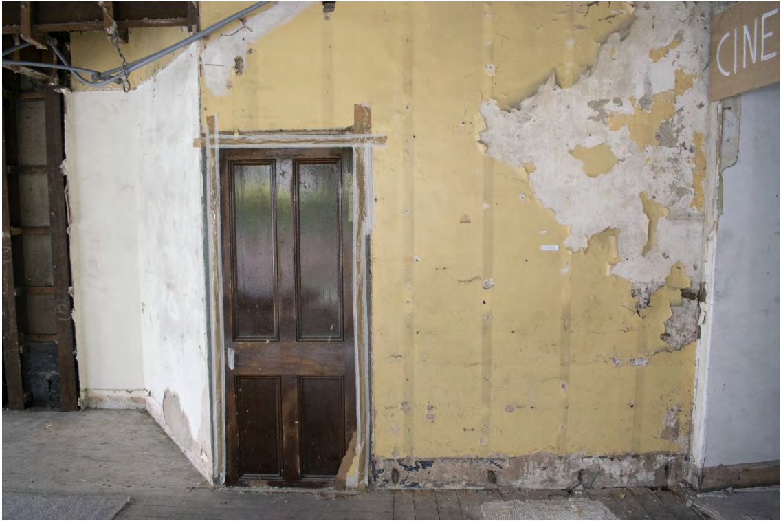
Plate 13 East wall with interior doorway and skirting board scarring.
