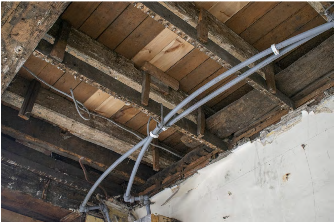
Plate 22 Detail of lath-and-plaster hangers and deterioration of plank ends.
