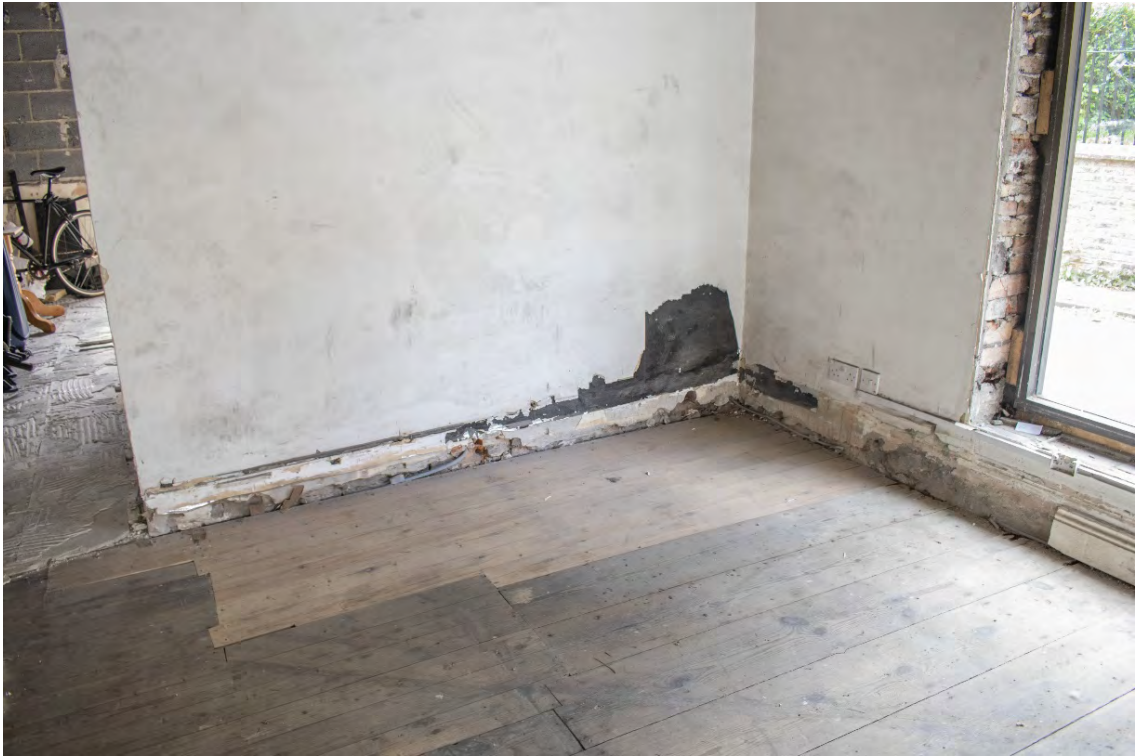
Plate 17 Floor alteration and subsidence.
