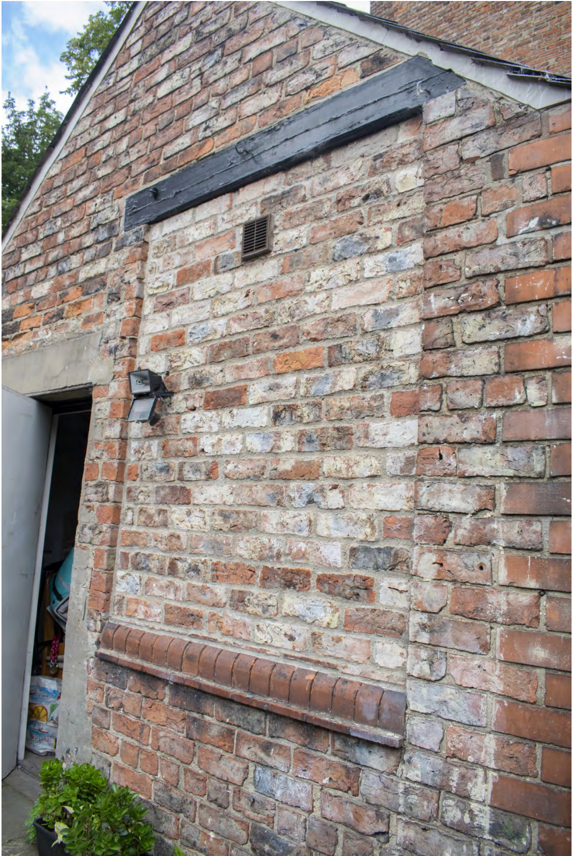
Plate 7 Infilled window in the rear extension.
