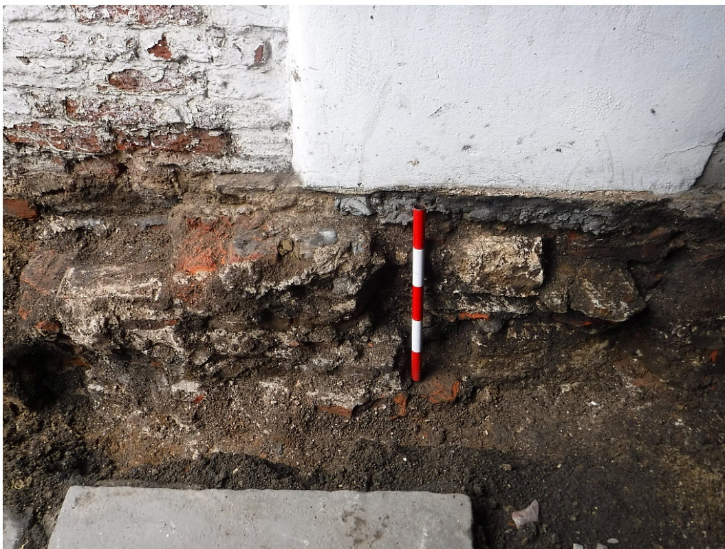
Plate 2 Foundations left and right of scale bar, facing west-south-west, scale unit 100mm
