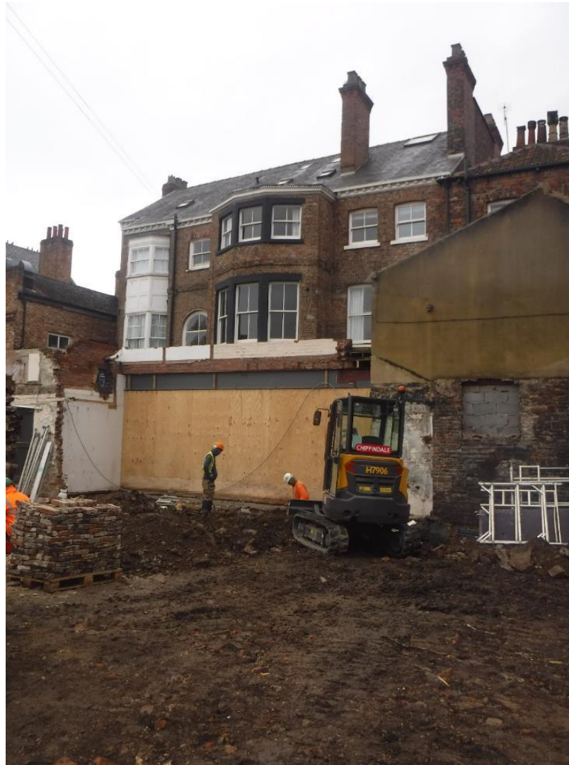
Plate 4 General view of Watching Brief at the rear of 27 Bootham area from the east
