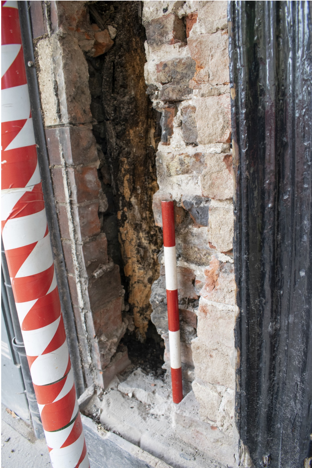
Plate 4 Base of timber post with wood worm deterioration.
