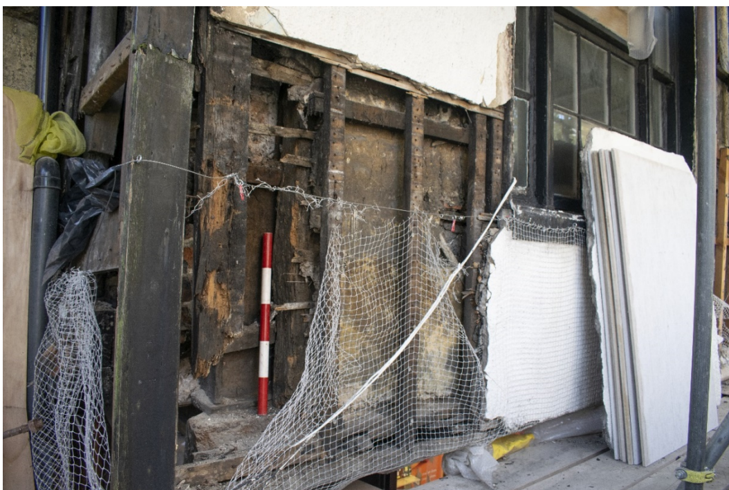
Plate 8 Deteriorated planks on left side of jetty.
