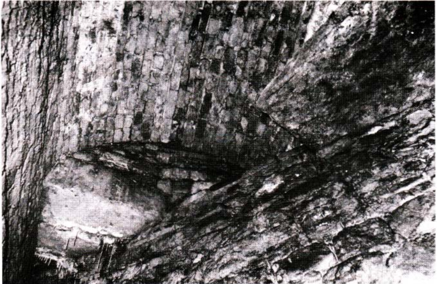
Tower 13: inside view of Victorian reconstruction of the angle in the defences immediately adjacent to Tofts Tower:- the brick vault and it's supports.
