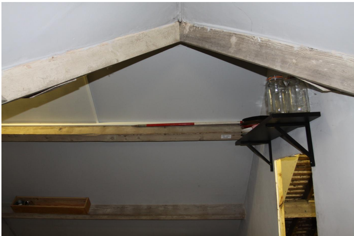
Plate 28 View of the ceiling within north-eastern upstairs room in Unit D, view south-east.
