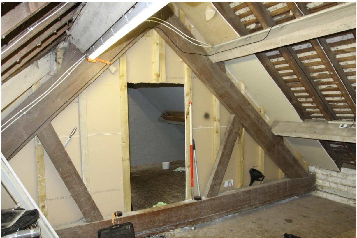
Plate 30 View of roof trusses within the south-western upstairs room in Unit D, view east.
