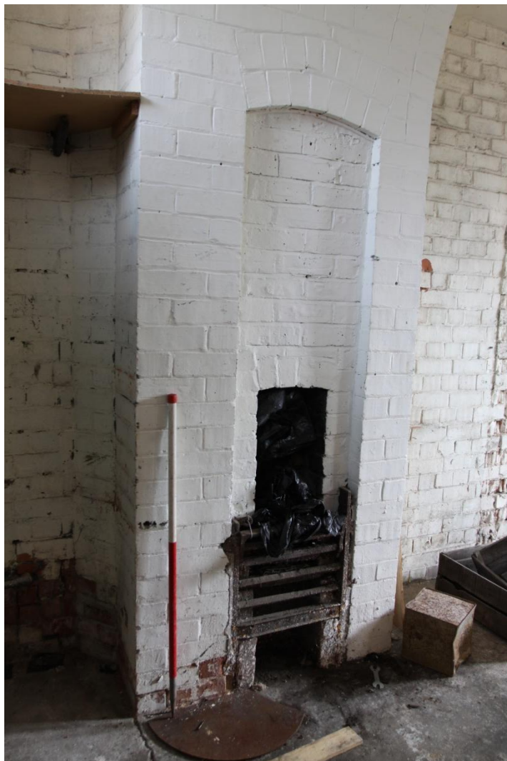
Plate 16 Detail of chimney and fireplace within north-eastern room of Unit B, view east.
