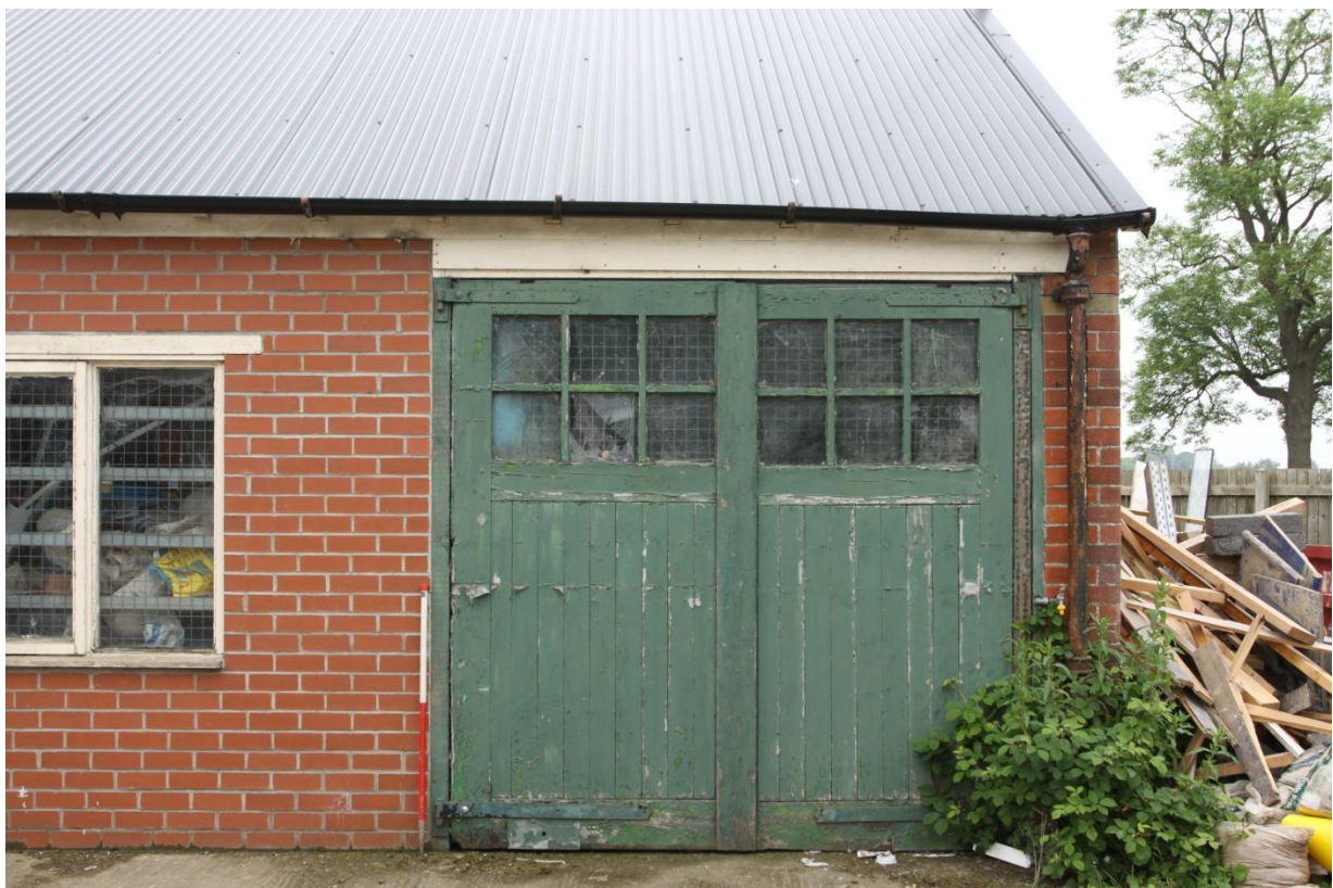
Plate 10 Double wooden doors in the north-eastern elevation of Unit A, view south-west.
