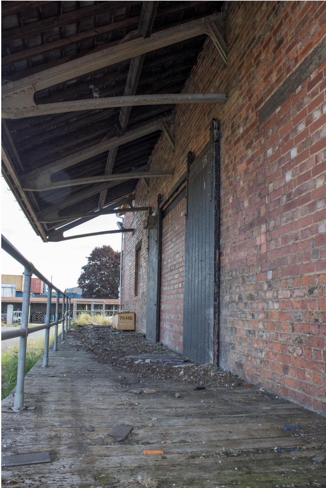
Plate 14: North elevation of the Locks Building showing raised platform and extending steel roof trusses for canopy
