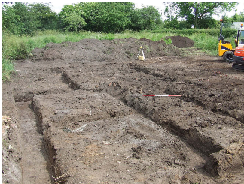
Plate 2 Overall view of surface strip and foundation trenches in northern 2/3rds of site
