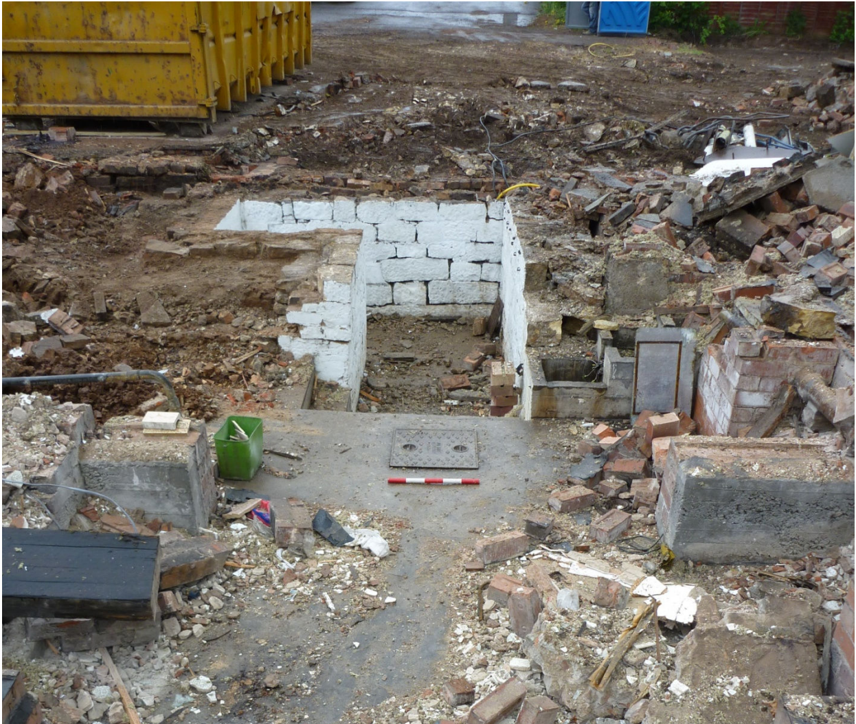
Plate 8 View of ice house entrance walls with ice house chamber access manhole in the foreground, looking north
