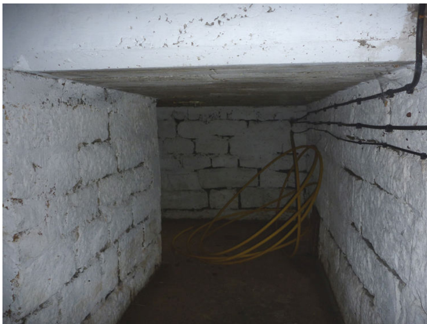
Plate 7 Interior view of ice house entrance prior to demolition of building above, looking north
