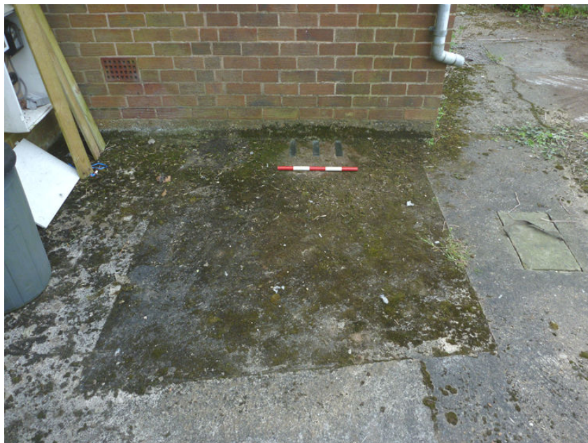
Plate 6 Concrete cap and sky-light over position of ice house entrance, looking west
