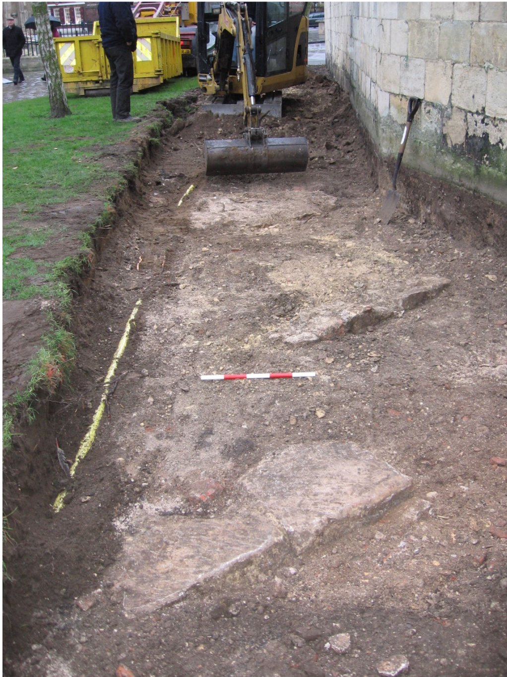
Plate 5 Contexts 8004 (foreground), 8005 (mid-ground), 8006 (adjacent to machine bucket), and services pipe 8007 (along the left hand side of the trench), scale unit 0.1m
