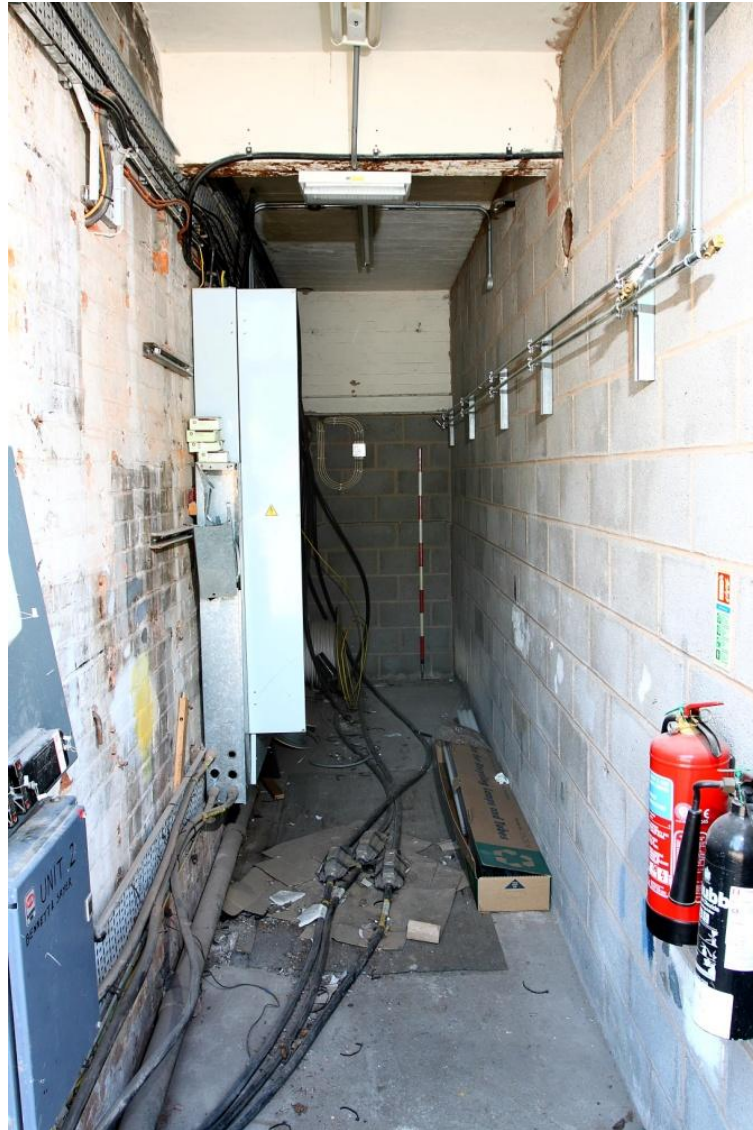
Plate 6 Electrical switch room, looking SW
