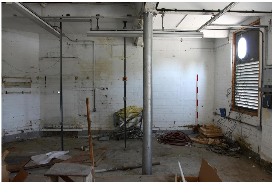
Plate 4 Plant room, looking NW
