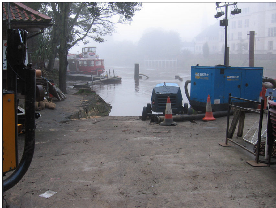
The coffer dam flooded, looking south-east
