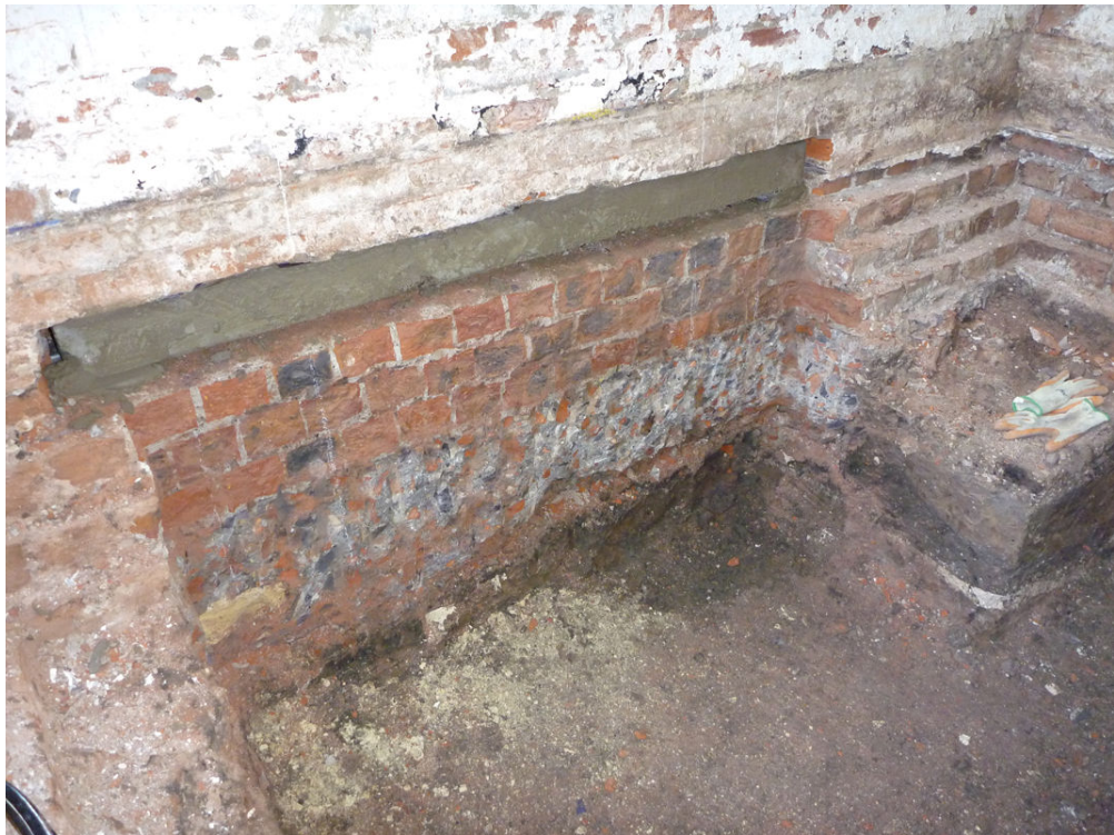
Plate 13 Foundation 1016 and 1020 beneath wall 1024, cut back for insertion of lintel in preparation for 2011 cabling works, looking north
