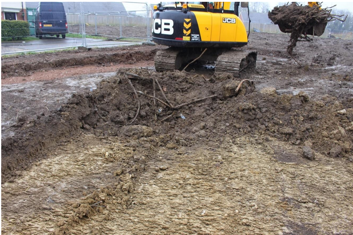
Plate 2: Excavation in progress across Roundhouse 2 (CG01) with modern waste material being removed
