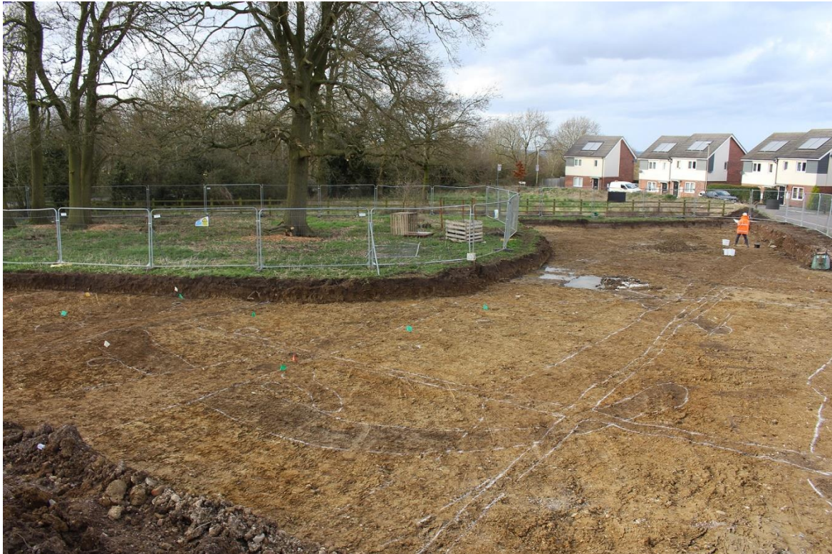
Plate 1: Excavation in progress with Roundhouse 9 (CG04) in foreground and the tree protection zone visible, facing north-west
