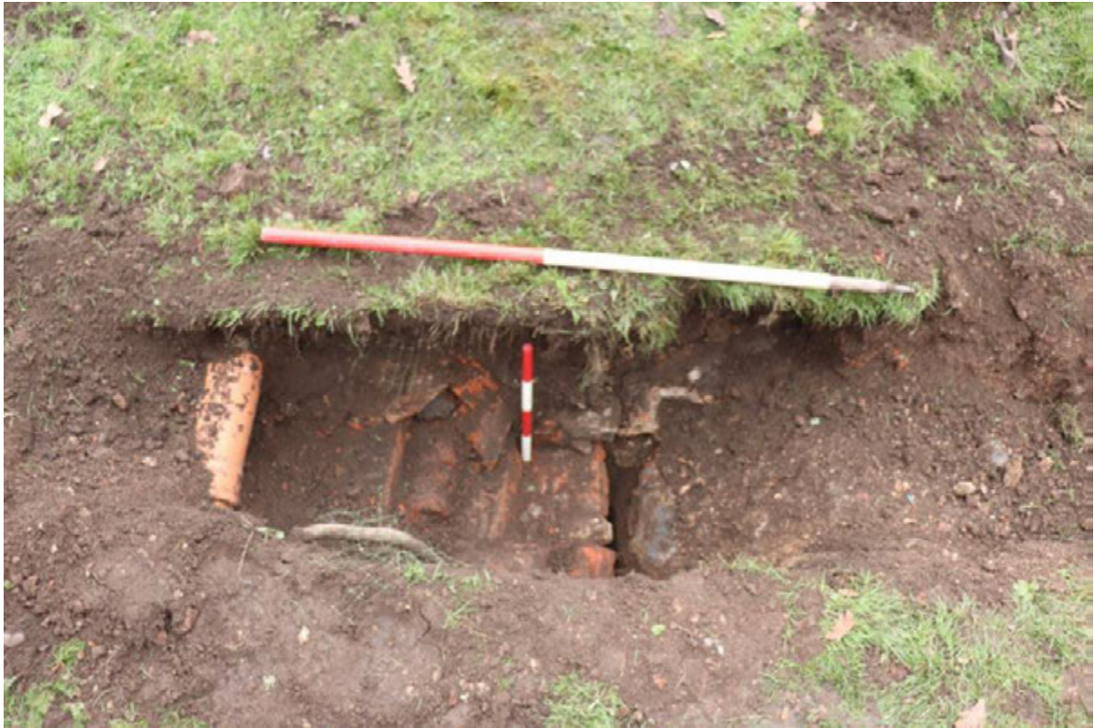
Plate 19: Top of culvert brick arch 1017, disturbed by modern services, on turfed slope at north-west edge of main excavation area, view south-east; 0.4m and 1m scales (initially exposed during the watching brief for the Biomass Boiler; WSM 77814; Arnold and Vaughan 2022)
