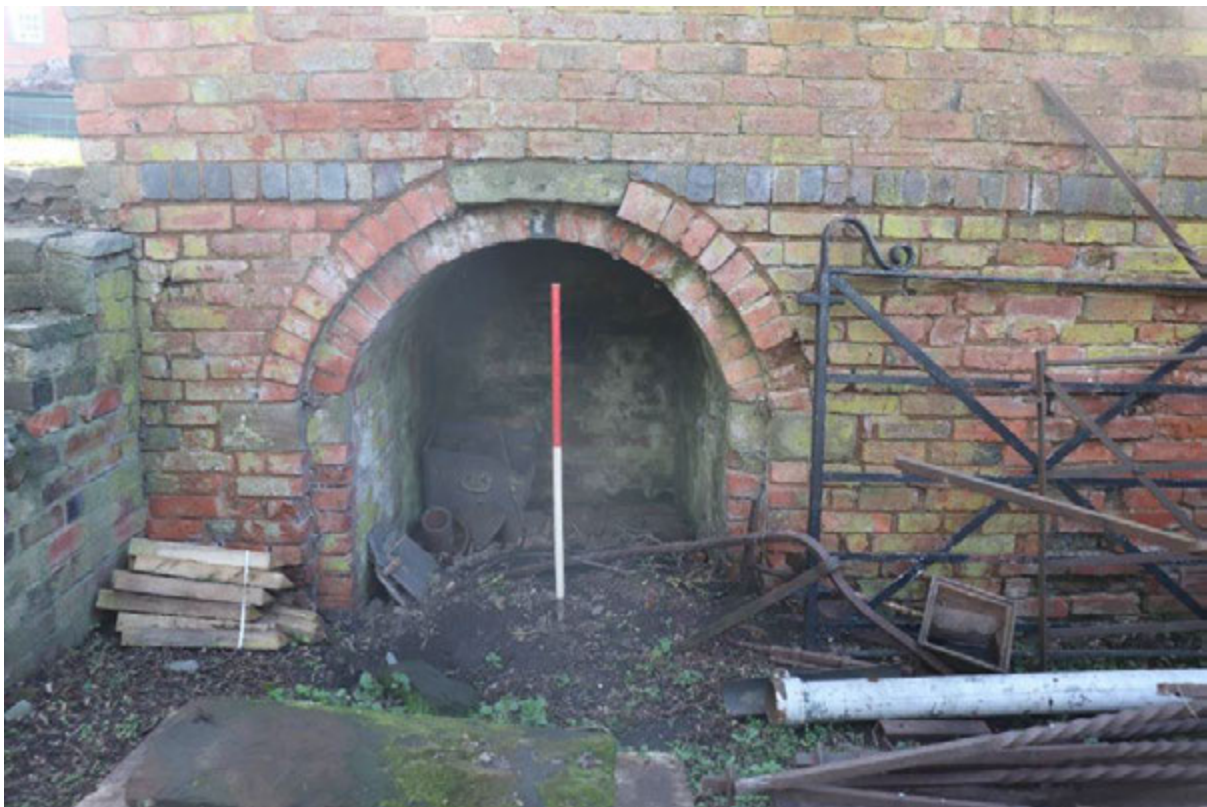
Plate 22: Blocked former outlet of brick culvert 1017 in Lower Yard to the north-west, view south-east; 1m scale
