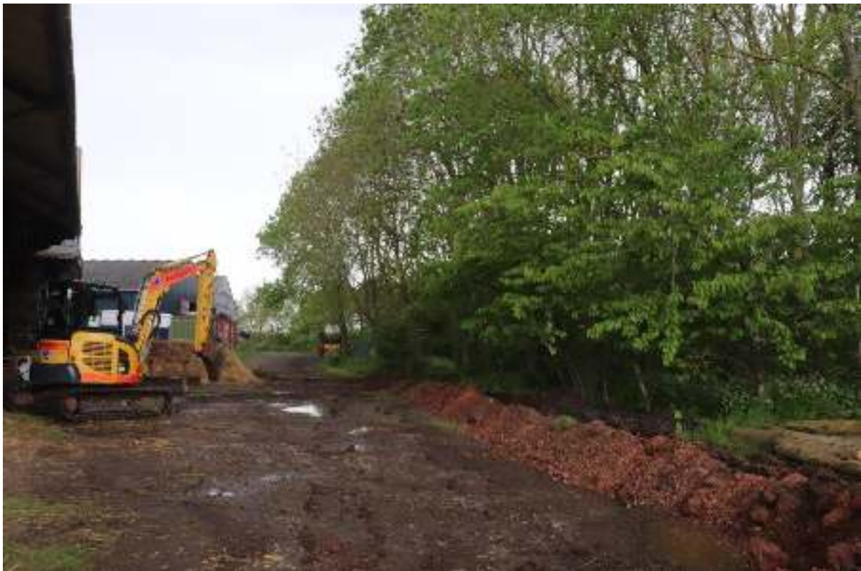
Plate 10: Trench along edge of farmyard and into the woodland, view north, no scales
