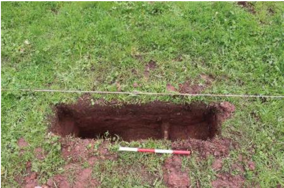
Plate 4: Existing water pipe to animal trough in line of trench, hand excavated, view east, 0.40m scale
