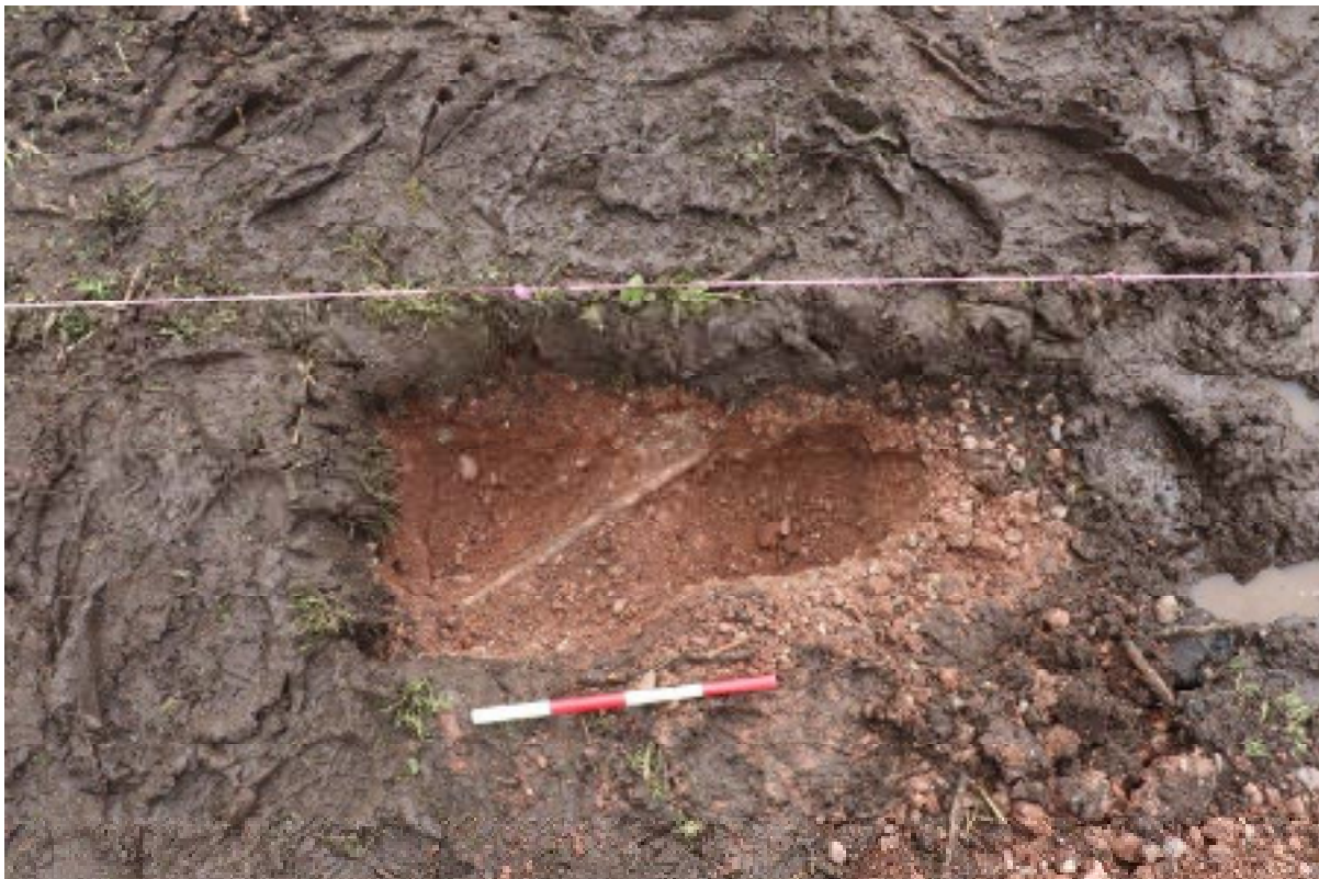
Plate 8: Existing water pipe crossing farmyard, hand excavated prior to works, 0.4m scale
