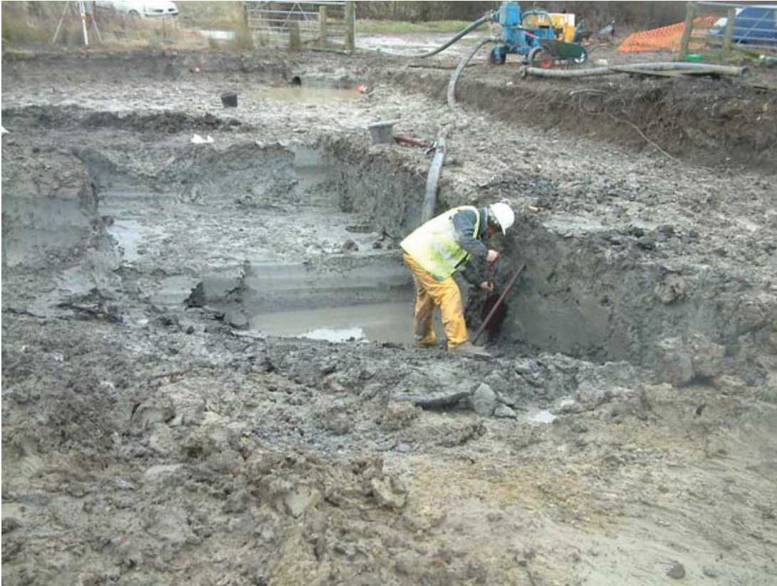
Figure 22 Excavating deep pond silts (view looking south over northern edge of pond)
