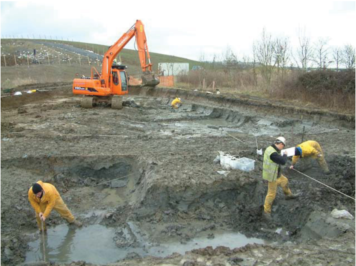
Figure 4 Pond (CG5) during excavation with fills exposed (pond edge viewed from west from front left to left of centre in background)
