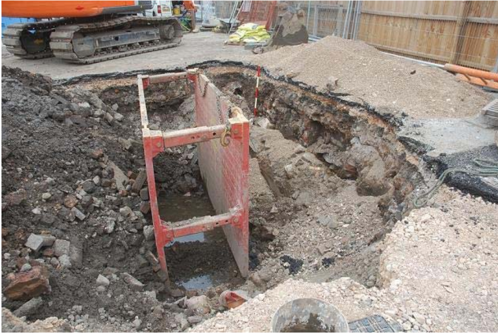
Plate 23 Cellar after walls removed showing made ground and modern services looking north west
