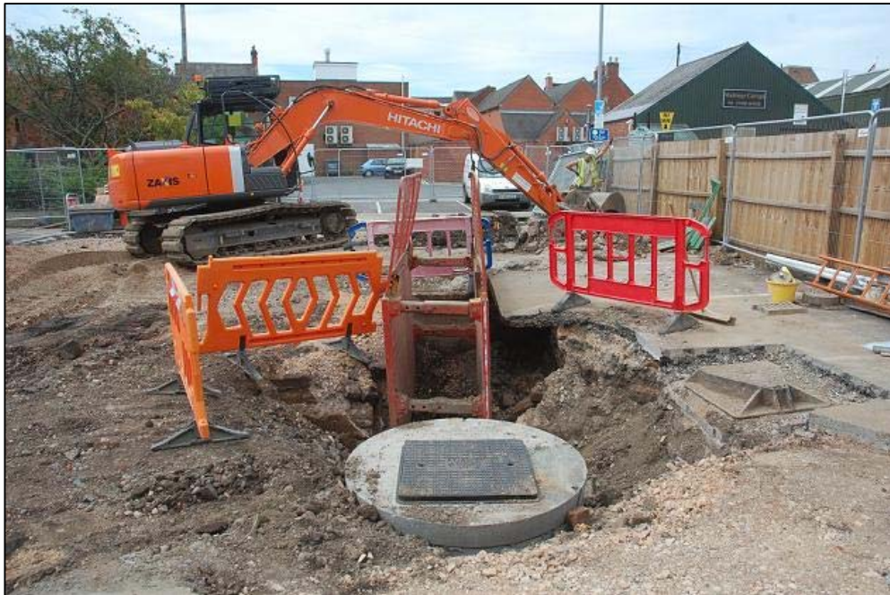
Plate 23 Phase 2 carpark being uncovered showing modern services, voids and brick wall of cellar looking South west
