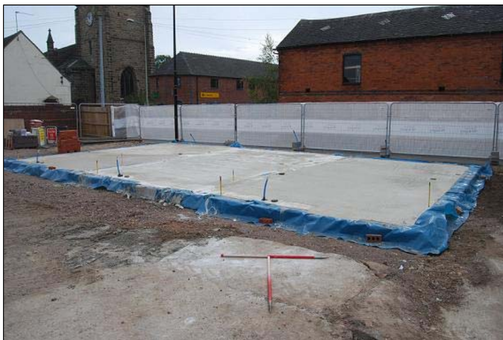
Plate 25 Concrete platform for houses after excavations were completed and all services had been installed looking southeast.
