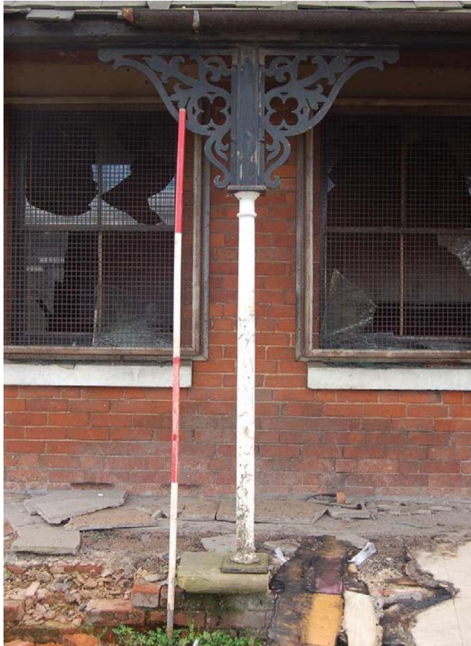
Plate 3. The public house, east wing, decorated iron pillar on north porch, view south
