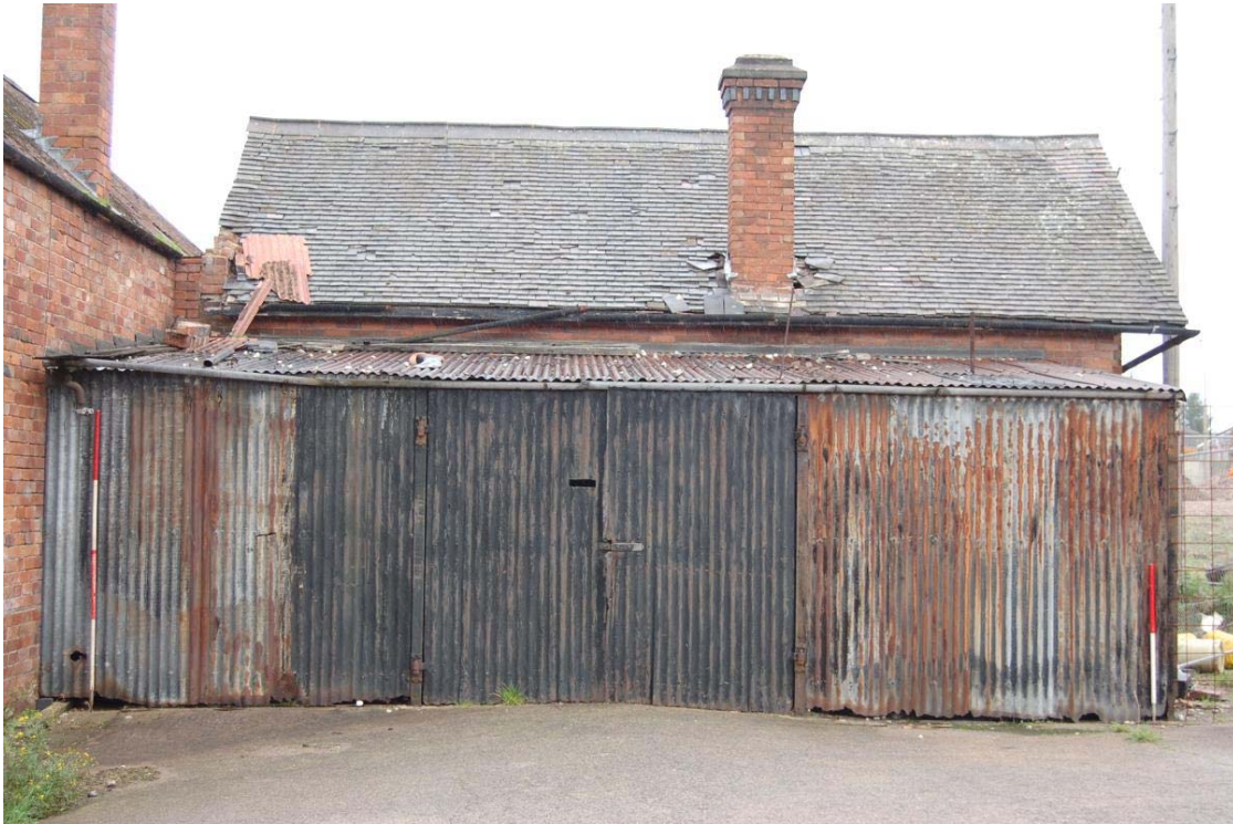
Plate 11. The public house, east wing and lean to, south elevations, view north
