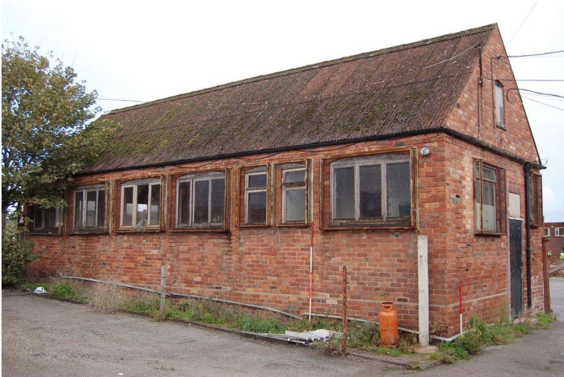
Plate 15. The public house, west wing, west and south elevations/gable end, view north-east
