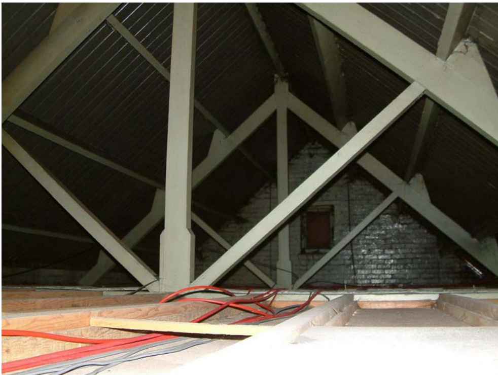
Plate 30. The public house, west wing, loft space and roof joists, view north
