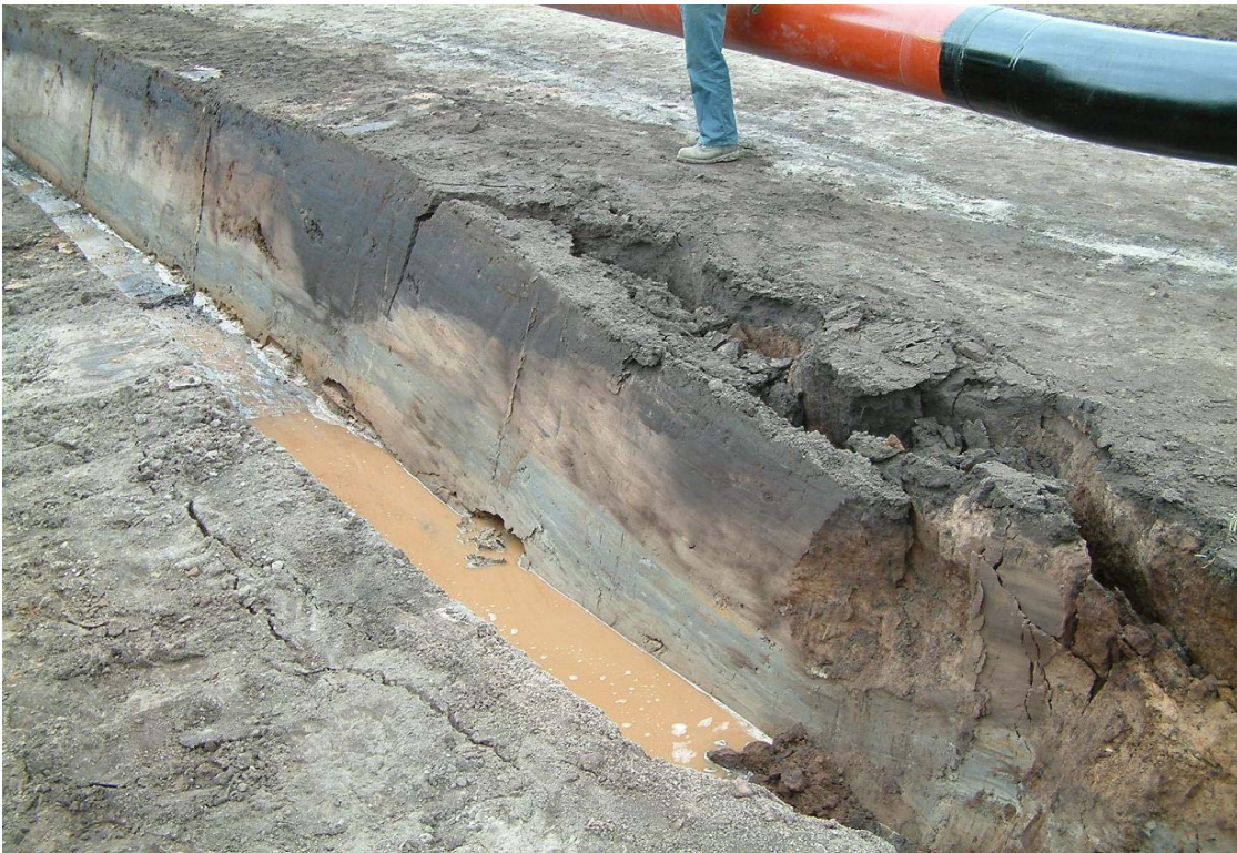
Plate 12: Organic deposits in field 4 reviled during excavation of the pipe trench, looking N
