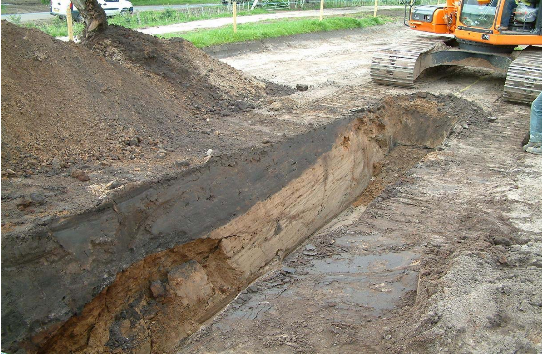
Plate 11: Organic deposits in field 4 reviled during excavation of the pipe trench, looking SW
