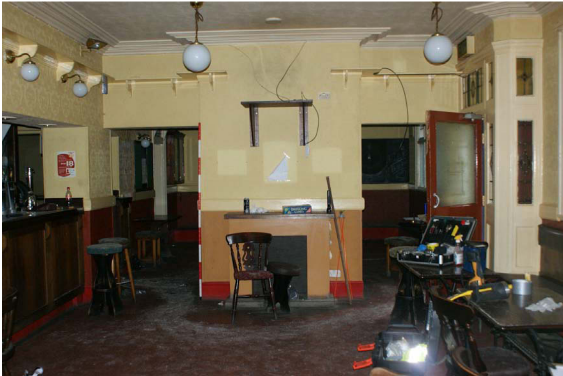
Plate 24: Fireplace in the bar with position of removed walls allowing access to former smoking room
