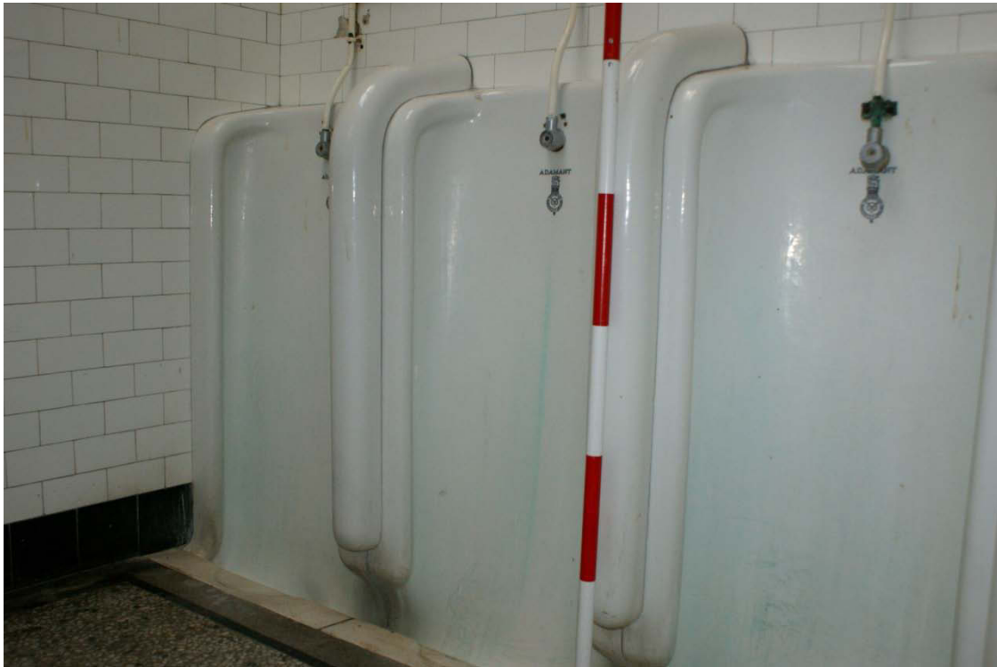
Plate 20: Row of 'Adamant' automatically flushing urinals
