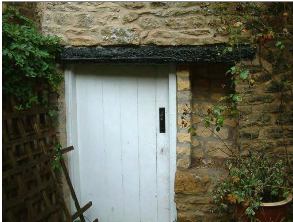
Plate 32: Blocked opening on southern elevation of shed to the rear of Kent House.
