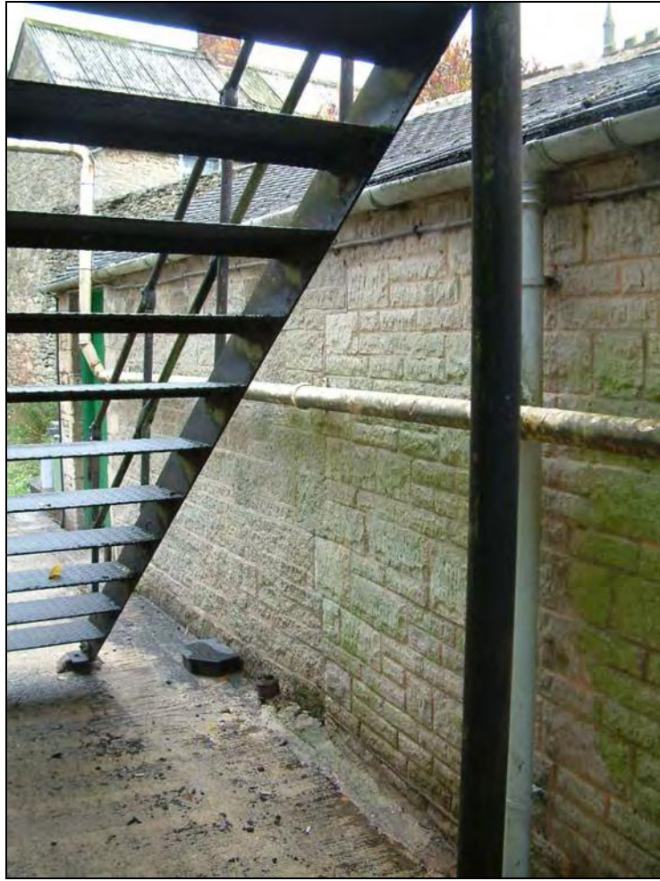
Plate 31: Building break in west elevation of sheds
